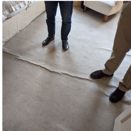
Photograph of Floor in 2 nd Floor Bedroom
