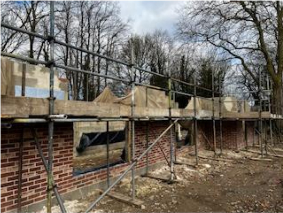
'Rear elevation' viewed from south. Trees in Church Lane and the site visible beyond
