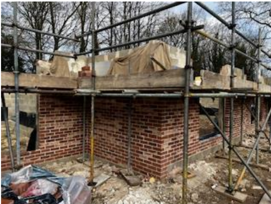
View from south-west towards a corner of the building on rear elevation, Church Lane beyond (north-east)
