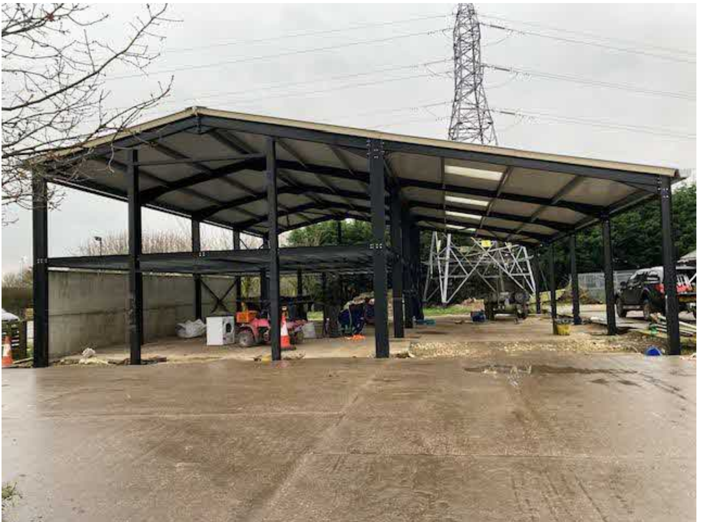
1. The front north east facing elevation of the framed equestrian building from the front concrete yard.
