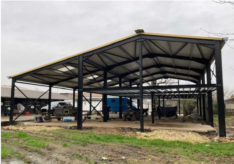
4. The rear south west elevation of the building with diagonal bracing in the rear bay.
