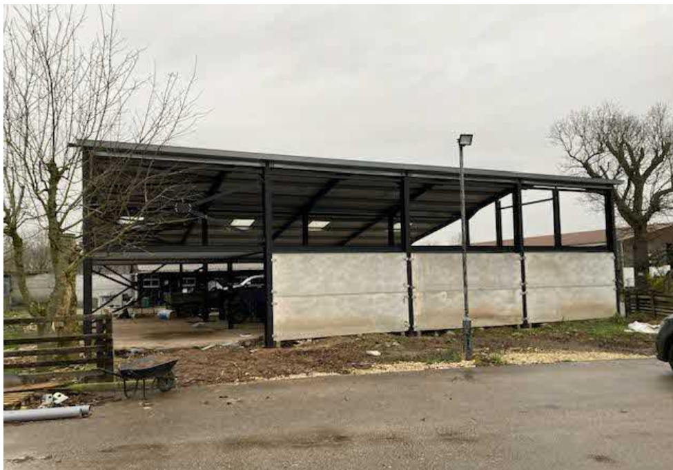
3. The south east side elevation of the building with concrete wall panels – from the car park.
