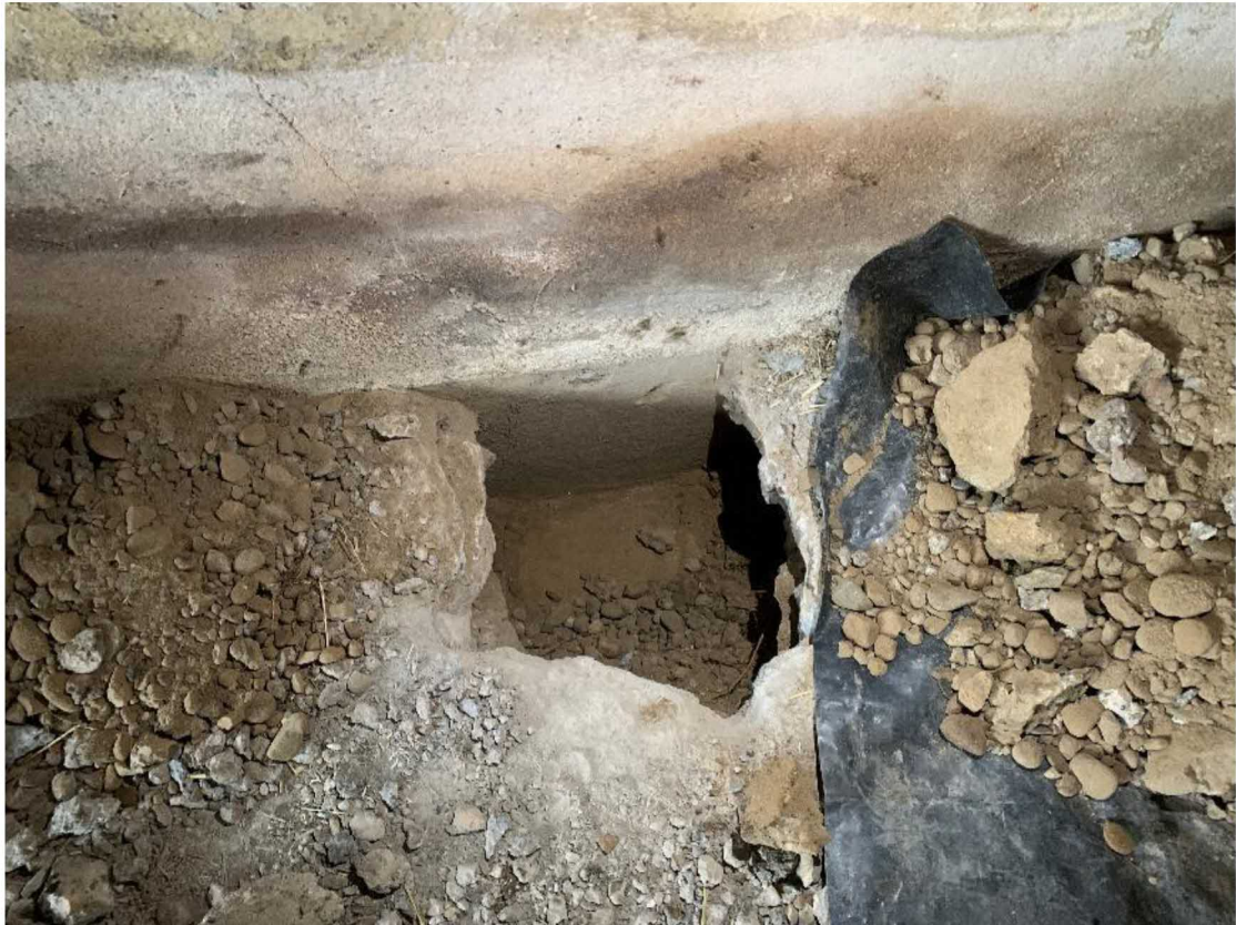
Photo 3: 23-10-2023 General view of the foundation pit in the larger building to the north east of the site (HP02).
