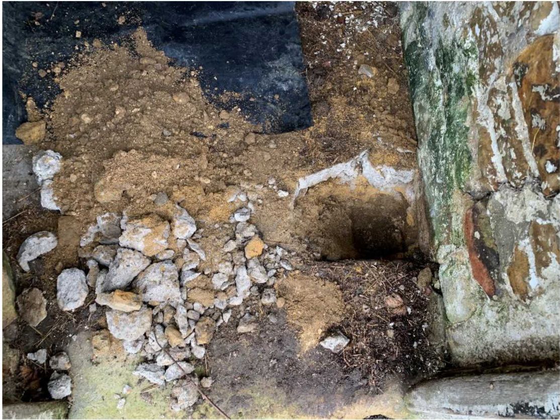
Photo 1: 23-10-2023 General view of the foundation pit in the small barn to the south west of the site (HP01).
