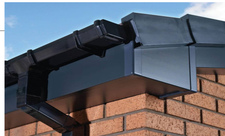
UPVC BLACK FASCIA AND SOFFIT WITH BLACK GUTTERING
