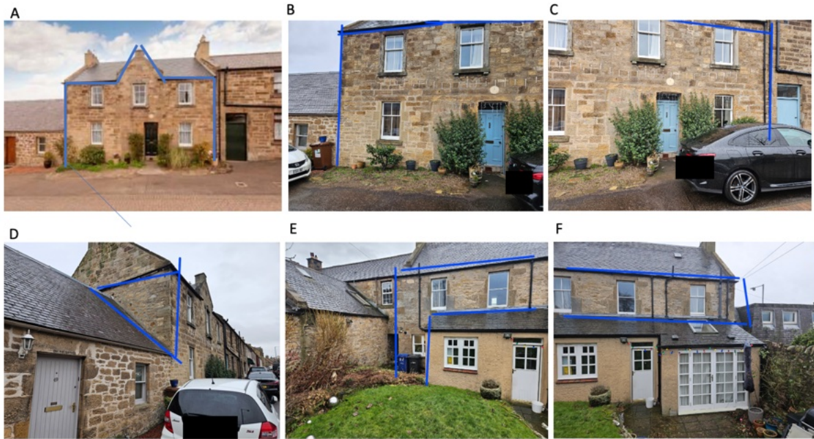
Figure 1: Areas of the house that require re-pointing. (A-C) Front elevation. (D) Left side of the house. Two equal triangular areas underneath the gutters require re-pointing, whereas the area above the gutters is correctly pointed with limestone mortar. (E-F) Back elevation. The extension does not require re-pointing.
