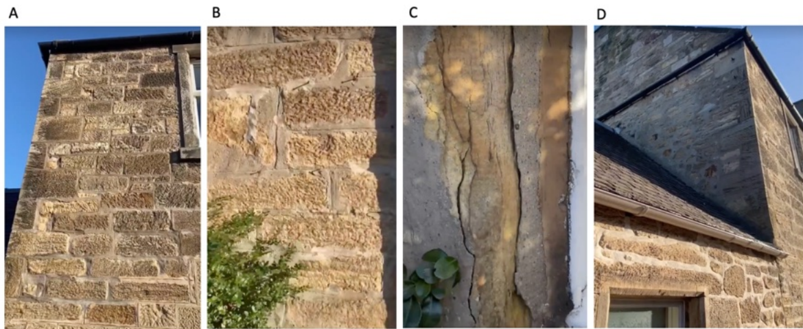
Figure 2: Concrete pointings. (A-D) Very wide concrete pointings that in some areas cover the sandstone and in others are severely cracked.
