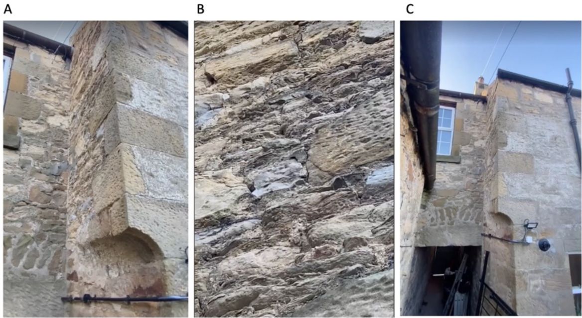
Figure 5: In certain areas, the stones are eroded and need to be repaired (A-C). C shows the entry of the Vennel that also requires re-pointing.
