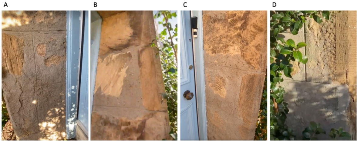
Figure 3: In several areas, the concrete covers whole stones which is for example apparent around the entrance door (A-D).
