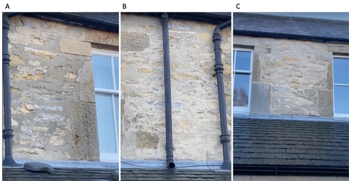
Figure 4: The rear elevation shows very wide concrete pointings that in areas cover considerable proportions of the sandstone.
