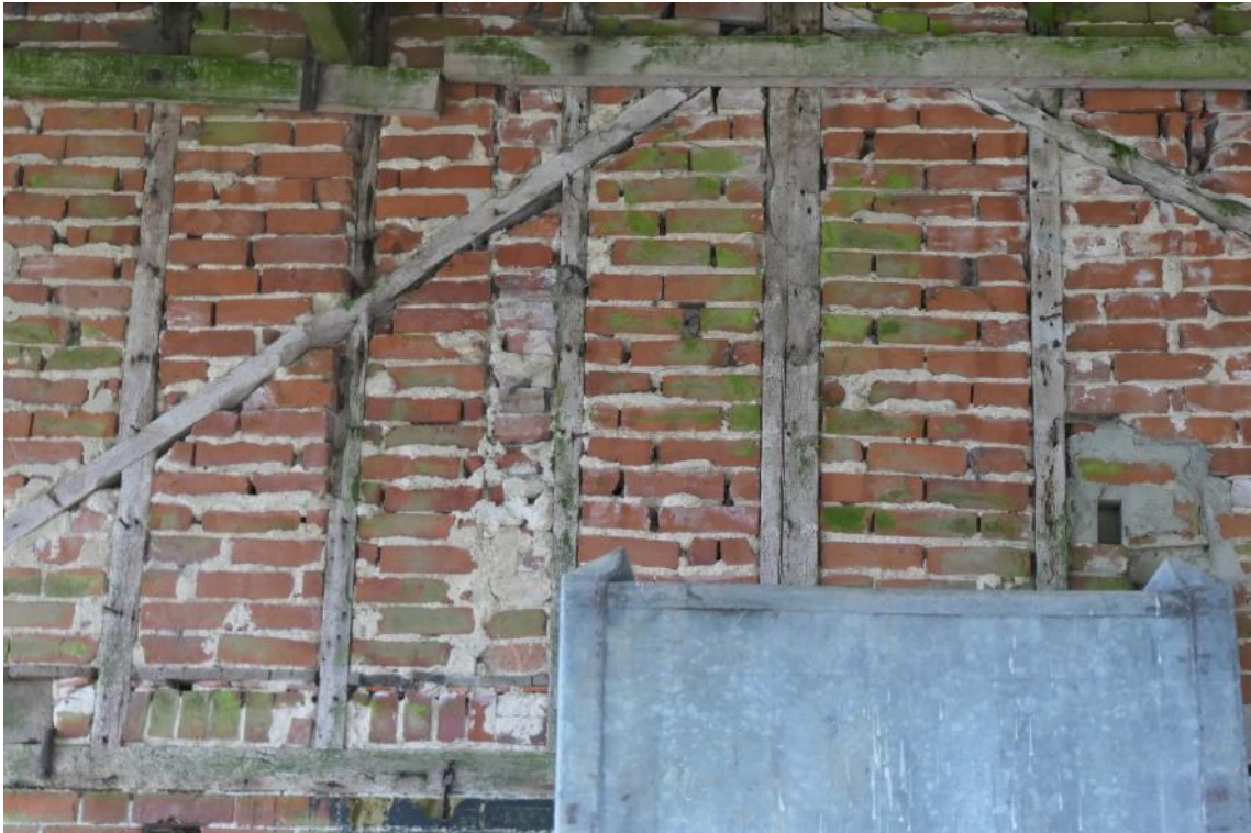
Photo 28 , gaps in brickwork which could offer suitable roosting opportunities on the western external wall of building three, looking east.
