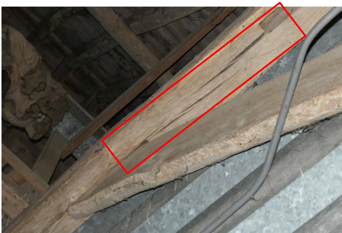
Photo 13 , mortis and tenon joint and crack in beam highlighted in red which offers suitable roosting locations.
