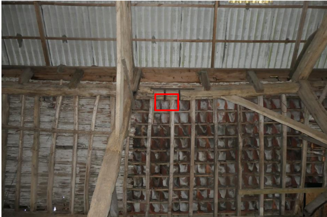
Photo 19 , roosting location of Pipistrelle sp., highlighted in red along the eastern aspect of building two.
