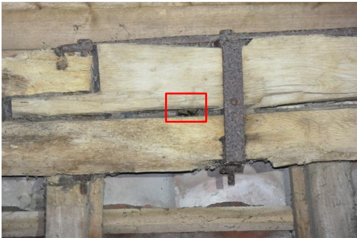
Photo 18 , Pipistrelle sp. highlighted in red roosting within a crack in a beam in building two.
