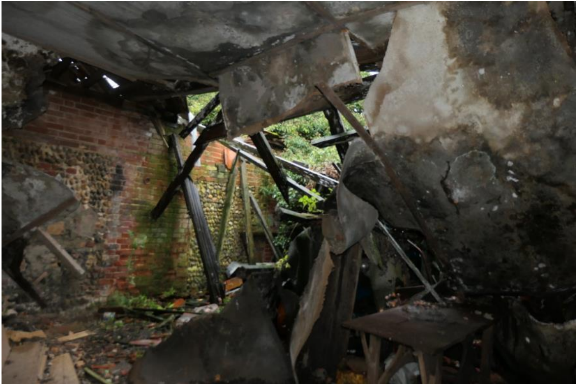
Photo 31 , internal view of the central section of the cart lodge with a collapsed roof, looking east.
