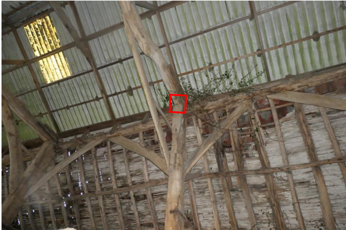
Photo 21 , roosting location of the Myotis sp., within a mortise and tenon joint along the western aspect of building two, highlighted in red.
