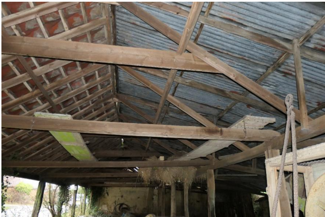
Photo 30 , internal view of the southern section of the cart lodge, looking north.
