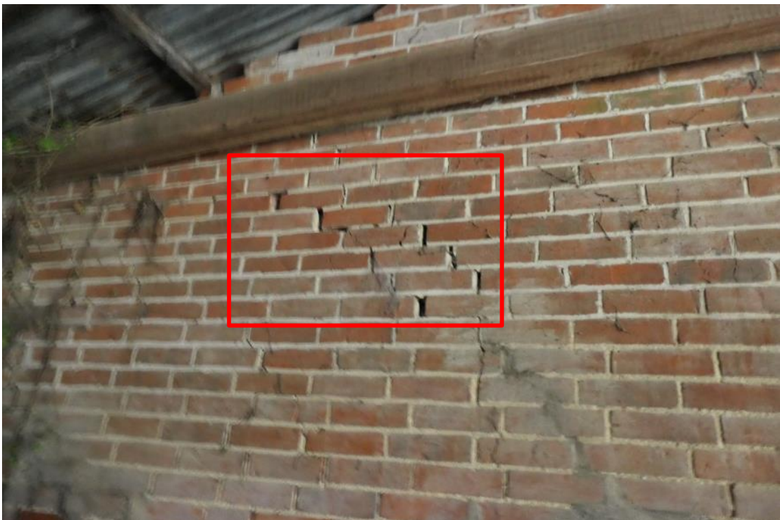
Photo 32 , cracks in brickwork which could offer suitable roosting opportunities, highlighted in red and looking south.
