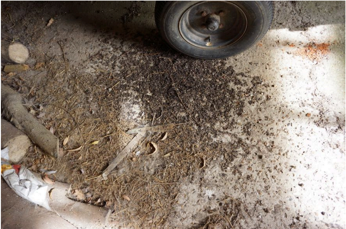
Photo 15 , internal view of the open barn, showing collection of bat droppings.
