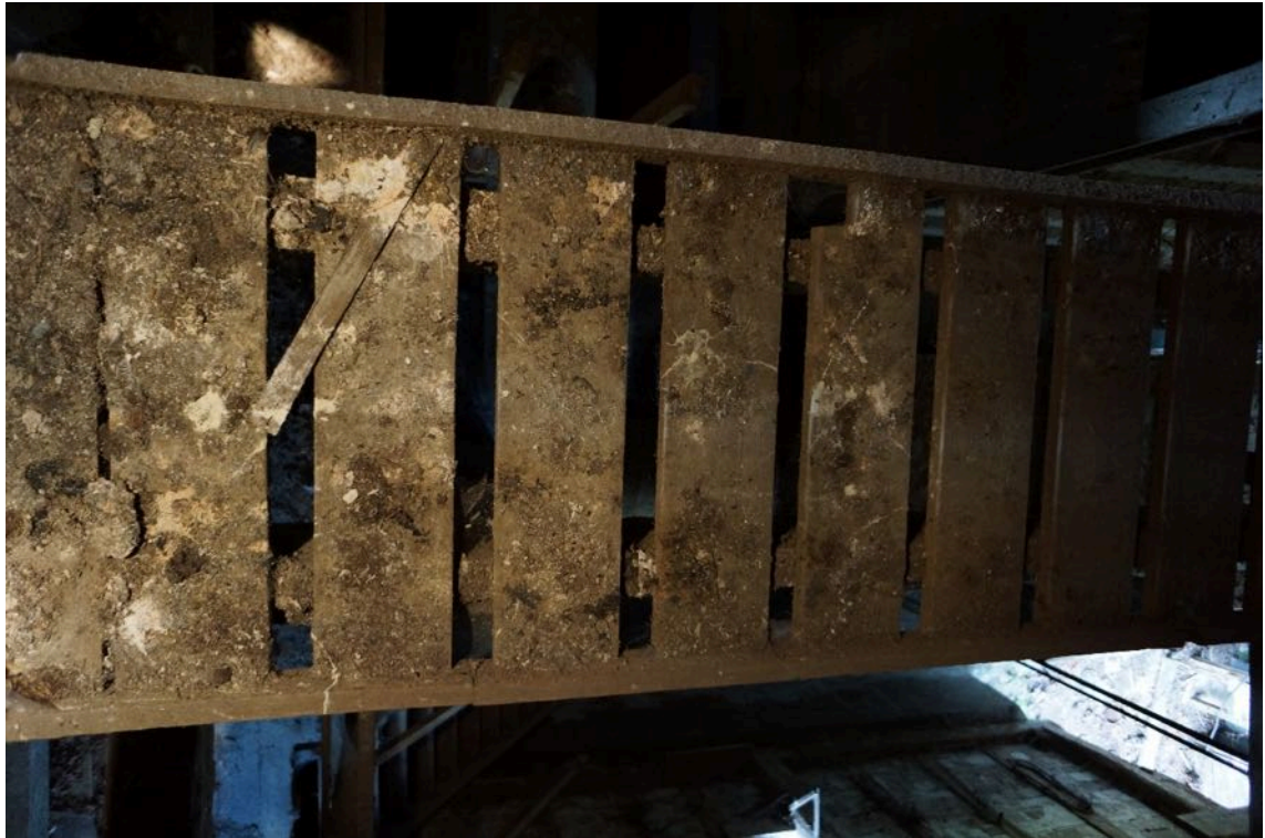
Photo 11 , internal view of the grain store, showing barn owl pellets/straining and scattered bat droppings.
