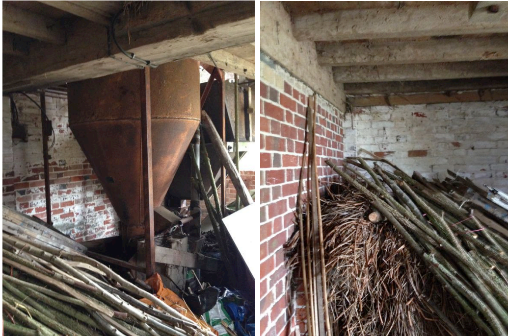
View of the oak floor structure with brick walls to the ground floor.
