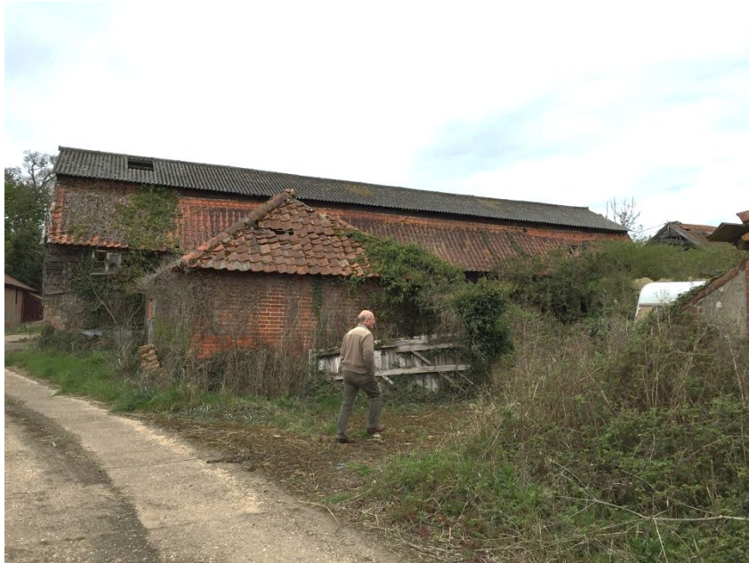
Image depicting the lowered central asbestos section of roof to be raised and the easterly wing.
