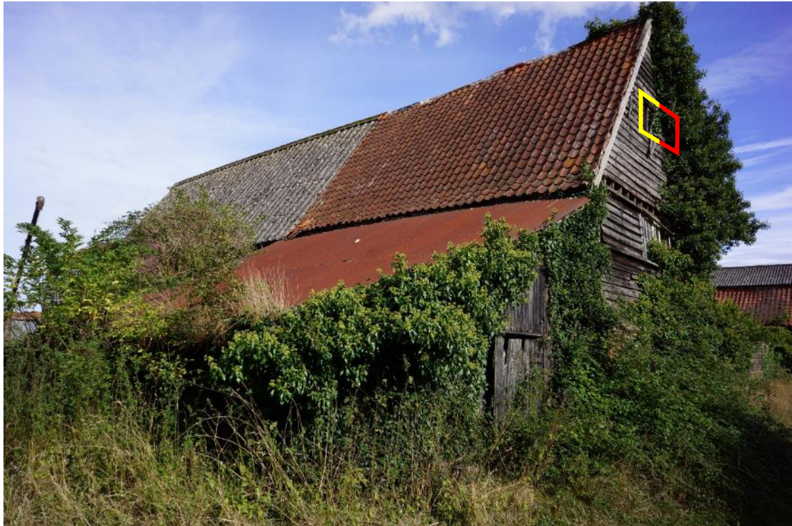
Photo 2 , common pipistrelle and brown long-eared access points on south gable end of building two (the grain store) highlighted in yellow and red respectively.
