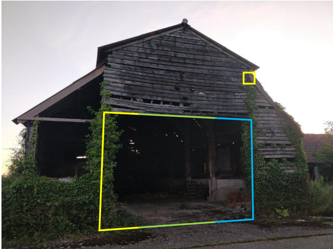
Photo 1 , common pipistrelle, barbastelle and Natterer's access points on south gable end of building three (the open barn) highlighted in yellow, green and blue respectively.
