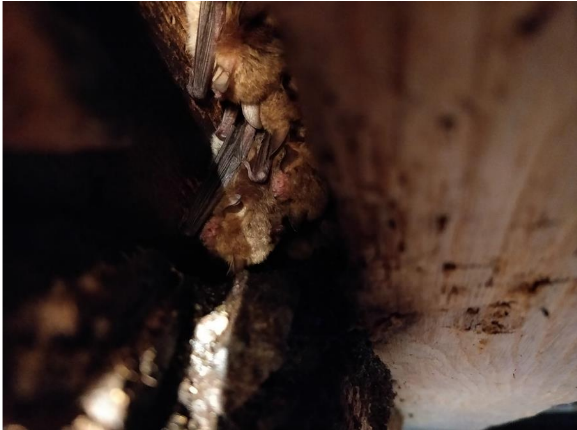
Photo 4 , Natterer's roosting within mortise and tenon joint in building three.
