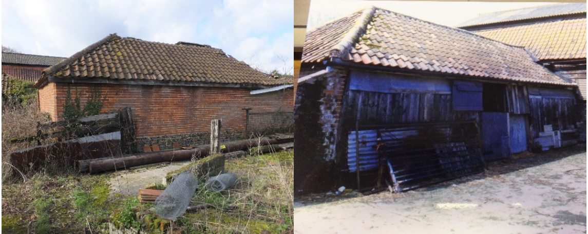
Low brick built piggery, possibly former stabling for heavy horses, forming south side to open courtyard.
