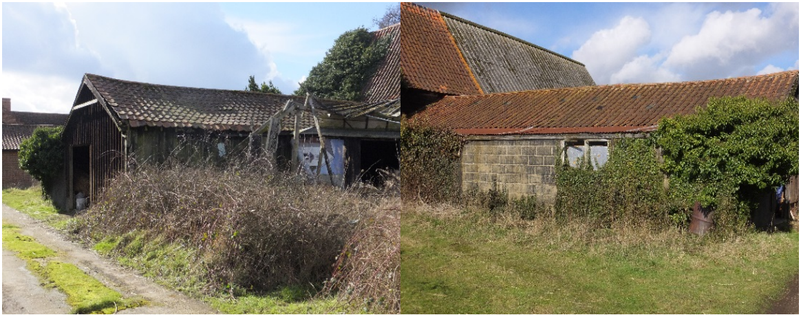
Timber framed construction, main axis east/west, with C20th extension to south, used for storage purposes.
