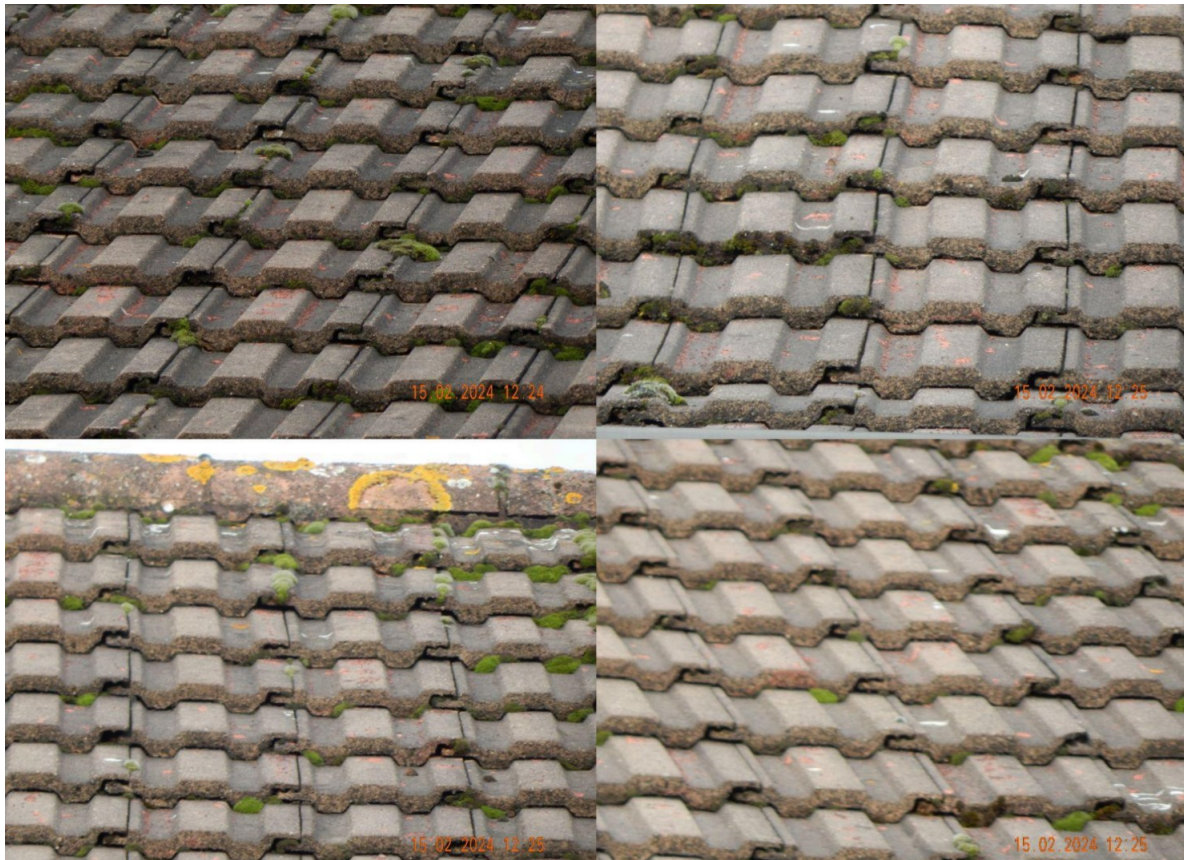
Image 3 – Close view of the main roof covering to show condition and lack of value to bats throughout
