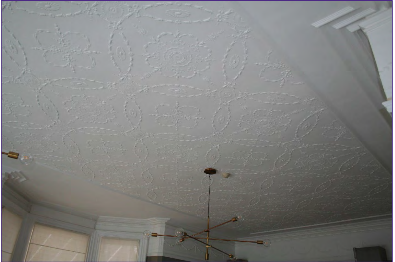
Plate 15: Textured ceiling paper and wall frieze in former drawing room (bar area).
