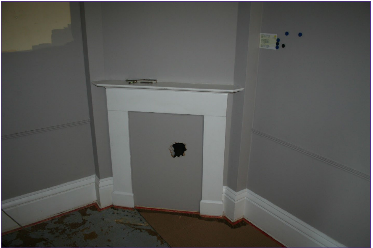
Plate 28: Remaining fire surround in first floor tower room.
