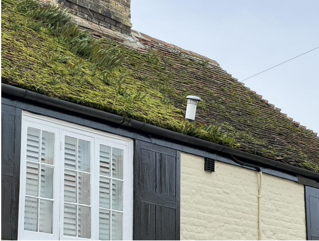
Photo (vi) – severe moss/plant growth to front elevation roof
