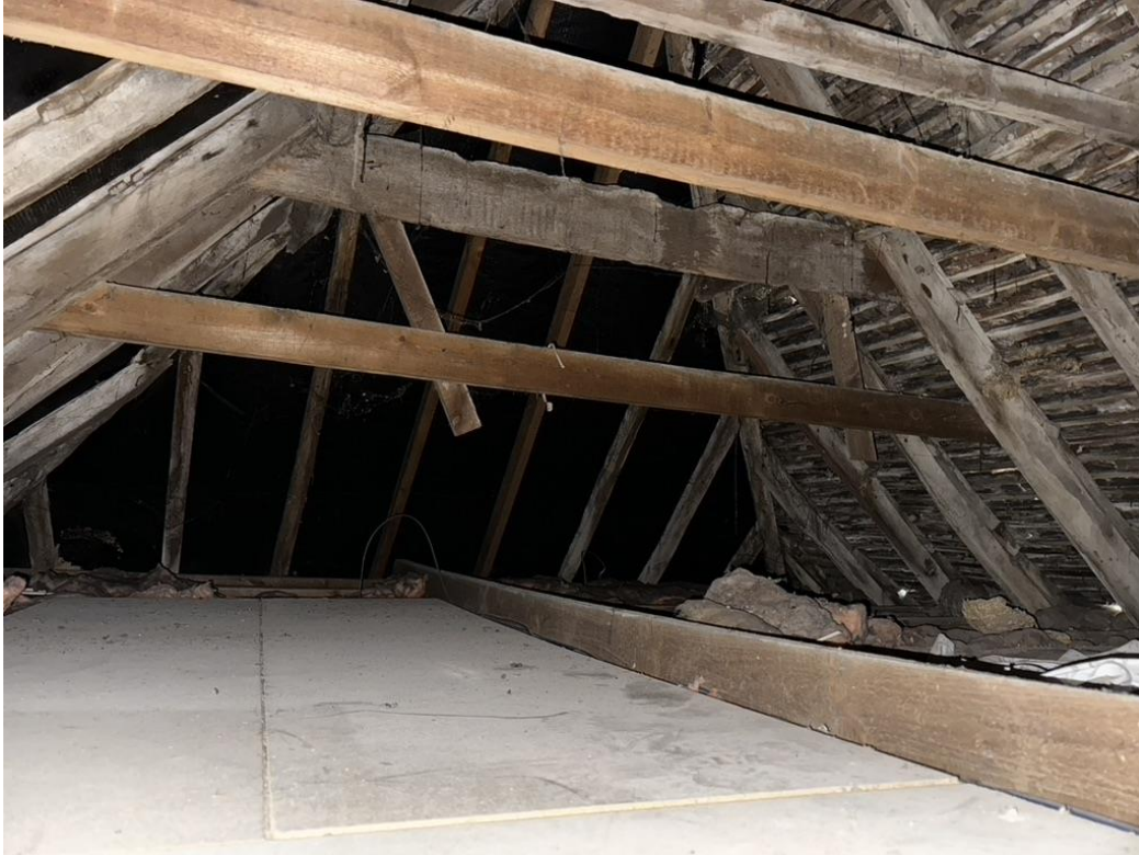
Photo (iv) – roof void showing rear and one gable having been recovered, with felt beneath
