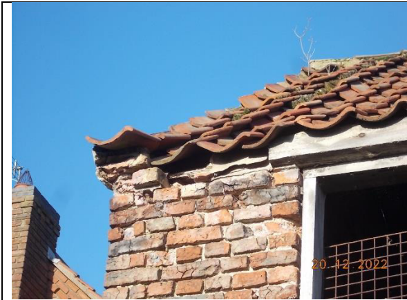
Plate 25: crevices between roof tiles.
