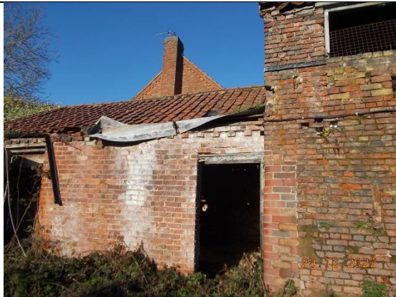
Plate 19: Building D, showing the clay pan-tiled roof. Photograph taken from the south.
