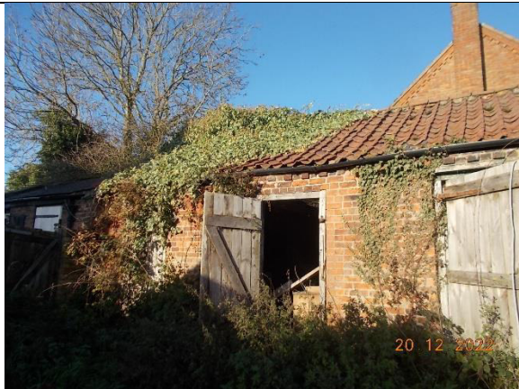
Plate 20: Building D, showing the ivy growing on the roof of the stall at the western end of the building. Photograph taken from the south.
