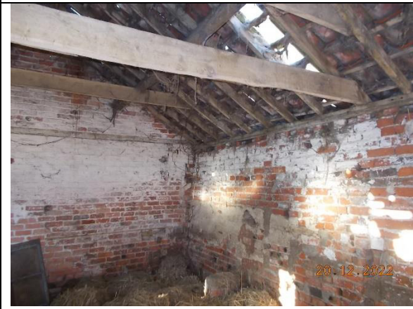
Plate 22: Building D, showing the interior timber frame at the eastern end of the building.
