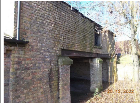
Plate 14: Building C, showing the open wall on the eastern side of the building. Photograph taken from the south-east.
