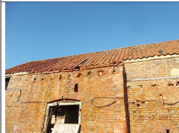
Plate 17: Building C, showing the clay pan-tiled roof of the eastern end of the building. Photograph taken from the south.
