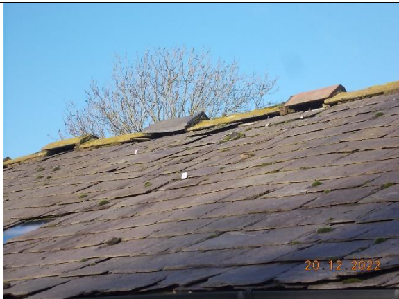
Plate 5: Building A, showing gaps beneath the ridge tiles.
