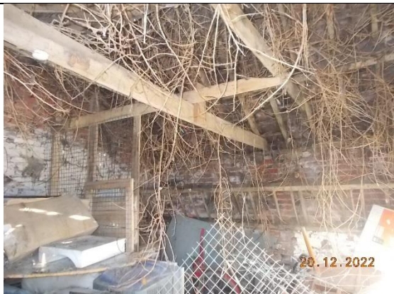
Plate 21: Building D, showing the ivy growing inside the stall.
