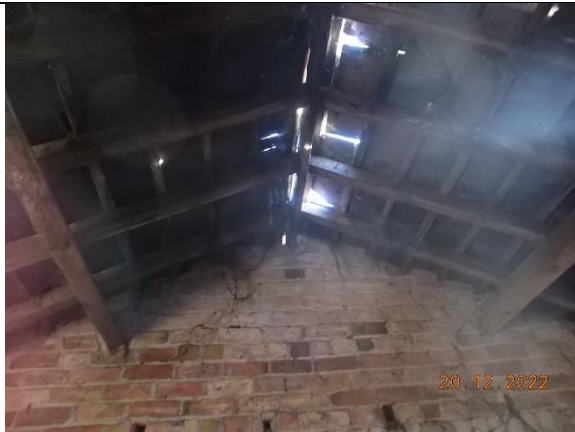
Plate 4: Building A, showing holes in the roof.
