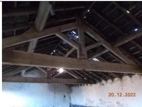
Plate 10: Building B, showing the holes in the roof.
