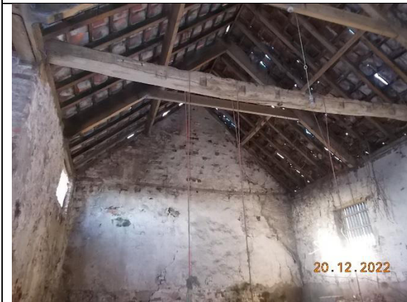
Plate 16: Building C, showing the room on the western end of the building.
