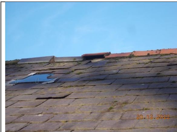
Plate 23: gaps beneath ridge tiles.
