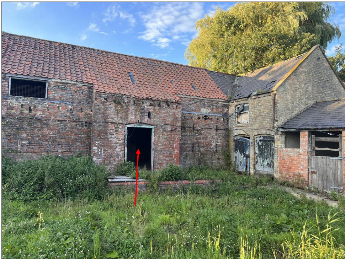
Photo 2: Access point for #R2 - common pipistrelle day roost (1 no.), #R4 - whiskered bat day roost (1 no.) and #R6 - brown long-eared bat day roost (2 no.)
