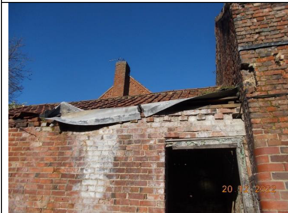
Plate 24: gaps beneath flashing.
