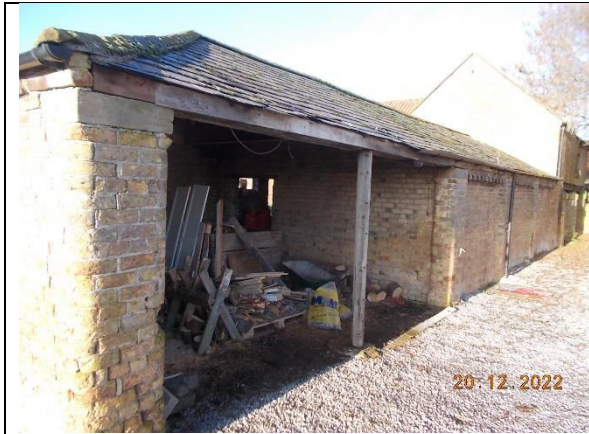
Plate 9: Building B, showing the open wall on the eastern side of the building. Photograph taken from the south-east.
