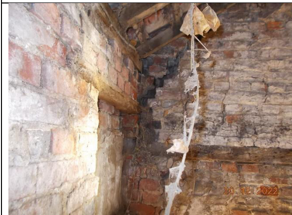
Plate 27: holes and deep cracks in brick walls.
