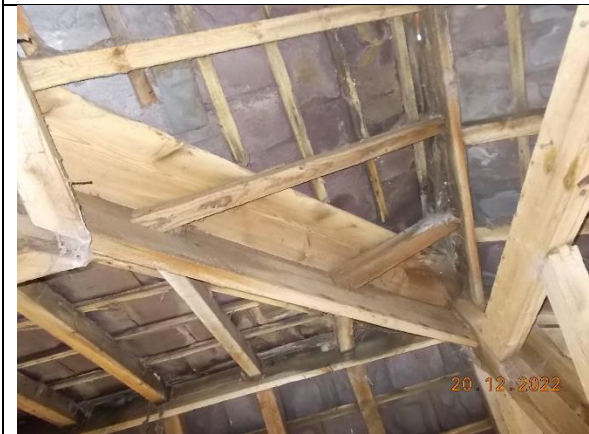
Plate 26: gaps between the internal timber framework and the roof tiles.
