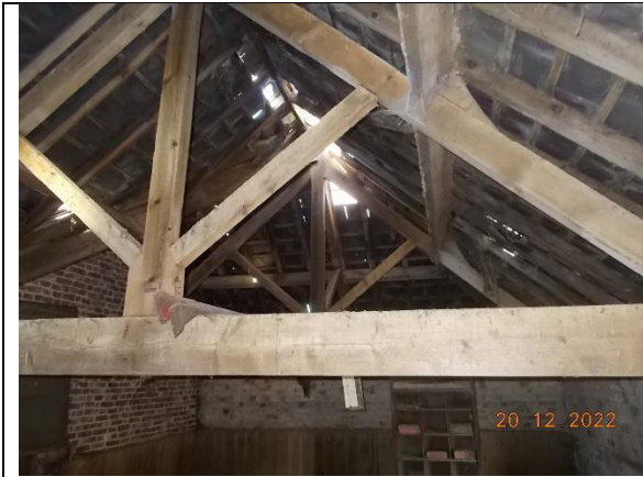
Plate 15: Building C, showing the timber frame and the slate-tiled roof of the 1 st floor room.
