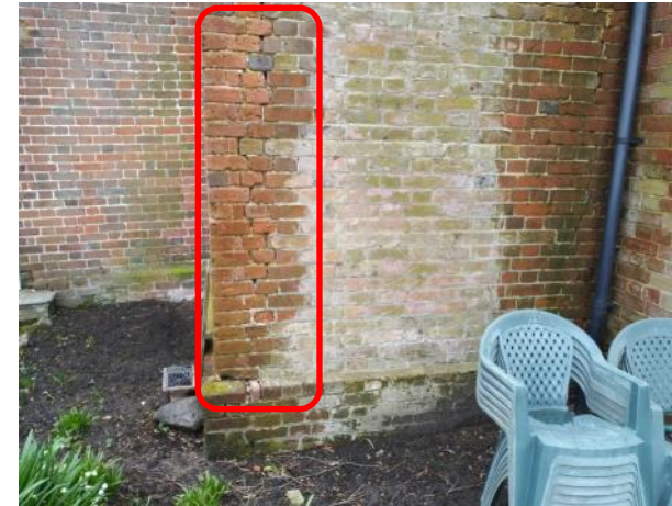
Figure 5.44: The brickwork to the western side of the Georgian stair core appears to have structural movement.
