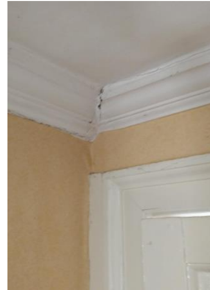
Figure 5.174: Showing the unevenness of the cornices to the room.
