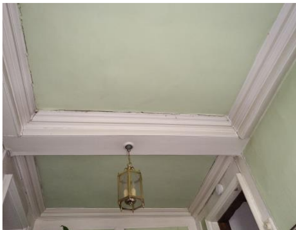
Figure 5.120: Showing the cornice to the ceiling and the cracking that is evident.
