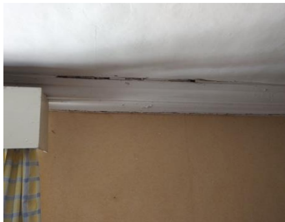
Figure 5.173: Showing the area of disrepair to the cornice on the southern wall.
