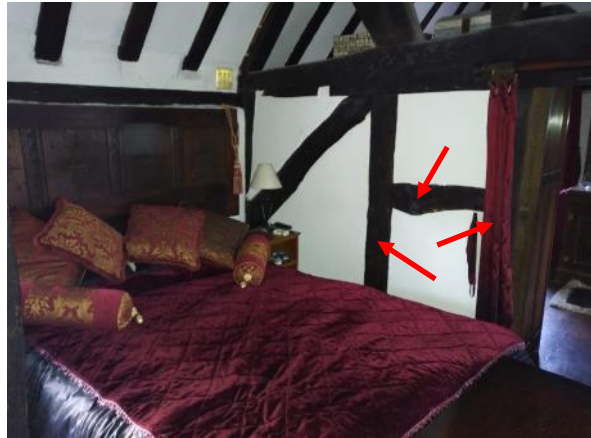
Figure 5.191: Showing the middle bay of the room (western side). The timber members added by the present owners are marked in red.
