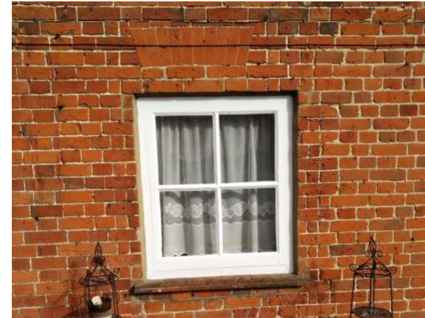
Figure 5.32: Showing the northern ground floor window to the Front Range's western elevation. Note how the window is wider than the head.
