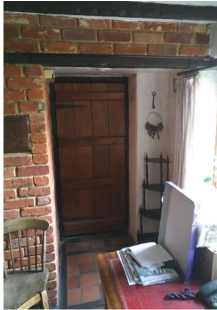
Figure 5.84: Showing the doorway from the Breakfast Room to the boiler room.
