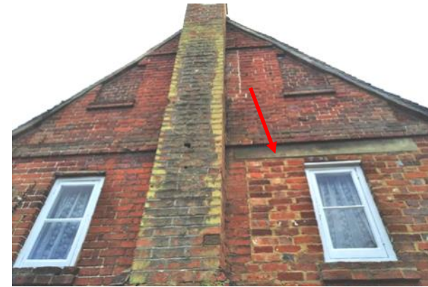
Figure 5.63: Showing the first floor of the Rear Range's northern elevation. Marked in red is the concrete lintel from a former window.
