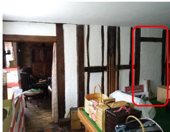
Figure 5.99: Showing the western wall of the Snooker Room. The former doorway into the Sitting Room is marked in red.
