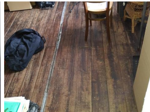
Figure 5.108: Showing the boarded floor to the Music Room and the portion of the floor that has partially subsided (right). Note the duct tape.
