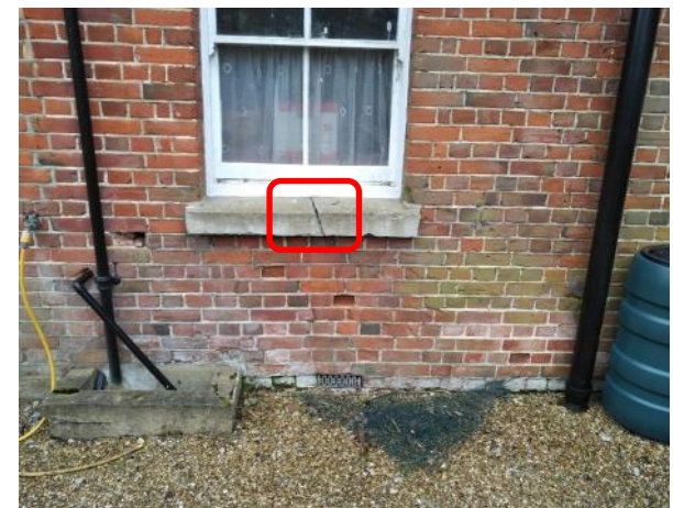
Figure 5.46: Showing the cracked concrete cill to the Victorian Extension's western ground floor window.
