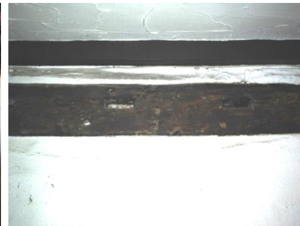
Figure 5.83: Showing the mortise joints for the previous lower ceiling joists in the Breakfast Room.
