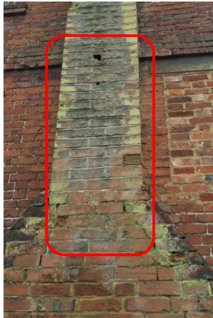
Figure 5.62: Showing the various cracks and holes to the northern chimneystack.
