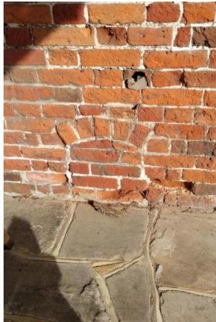
Figure 5.70: Showing a former opening at lower level in the Dining Room's western elevation.
