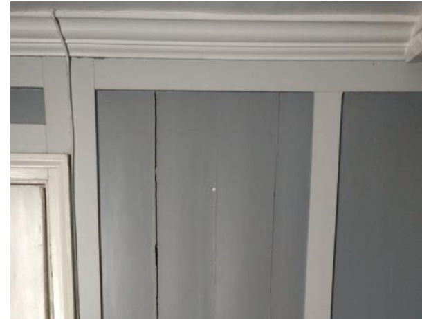
Figure 5.102: Showing a section of cracked panelling to the Music Room and a section of cornice above.
