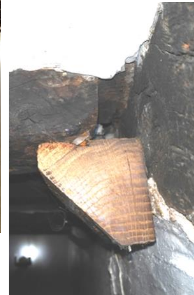
Figure 5.91: Showing how the joists to the Dining Room ceiling are dislocating from the joists.
