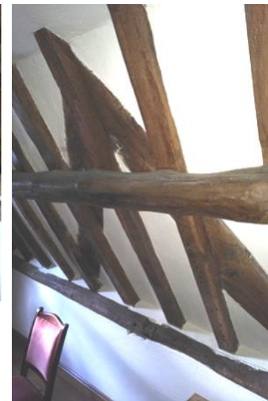
Figure 5.201: Showing the inverted V-shaped framing where the Rear Range's roof meets the Front Range.
