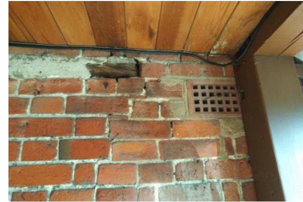
Figure 5.71: Showing part of the timber frame visible just below the covered walkway, on the Sitting Room's western elevation.
