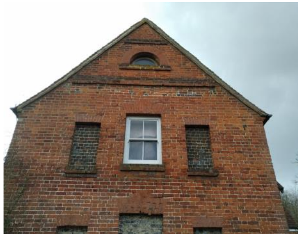
Figure 5.37: Showing the first floor and gable end of the Front Range's eastern elevation.
