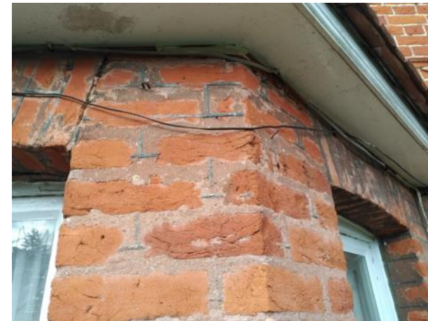
Figure 5.22: Showing evidence of tuck pointing on the Front Range's front elevation. The example shown lies on the canted bay window.
