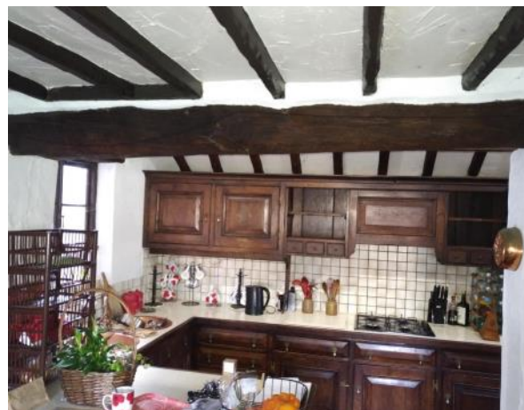
Figure 5.78: Showing the beam lintel to the opening between the Kitchen and Breakfast Room.
