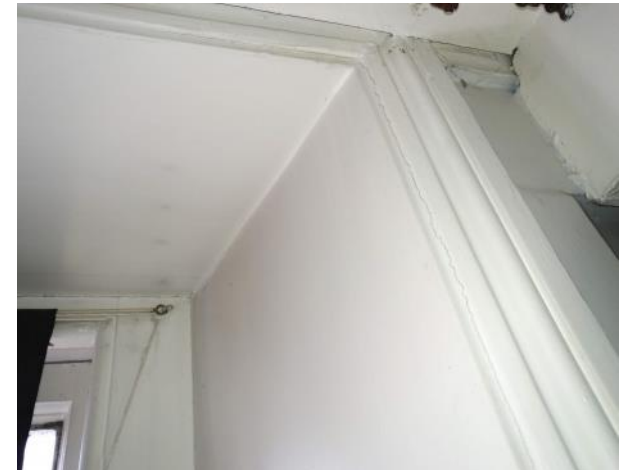
Figure 5.164: Showing how the eastern window's architrave is slightly truncated where it meets the ceiling.
