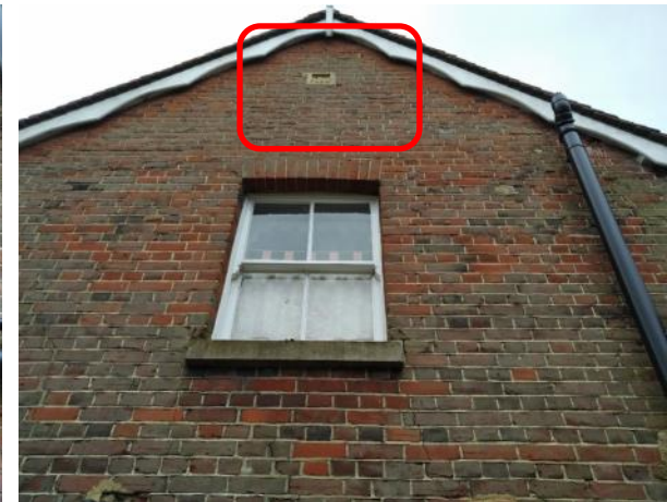
Figure 5.48: Showing the gable end of the Victorian Extension. The stone plaque’s location is marked in red.
