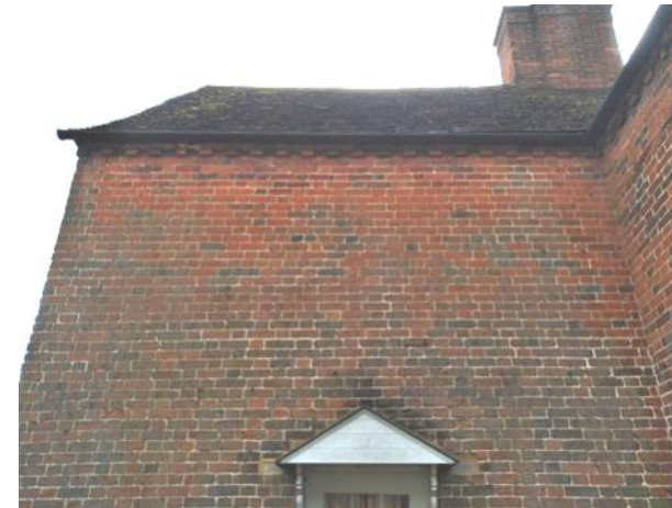
Figure 5.40: Showing the brick dentils to the western extreme of the Front Range's rear elevation.
