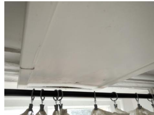
Figure 5.186: Showing how the central ceiling beam sits awkwardly against the western window's architrave.
