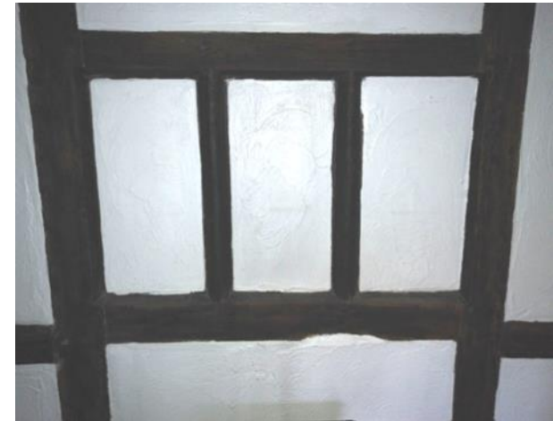
Figure 5.156: Showing the 17th century former window on the southern wall of the bathroom.
