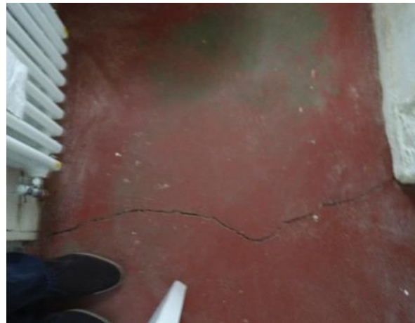
Figure 5.137: Showing the cracked concrete floor to the W.C..
