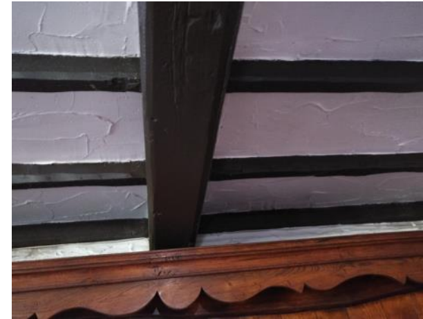
Figure 5.85: Showing the beam and joists on the Breakfast Room's ceiling and the unsympathetic plastering.
