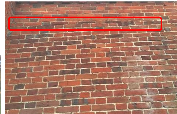
Figure 5.42: Showing the brick course on the stair core's eastern elevation that diminishes from a full height brick to nothing (marked in red).
