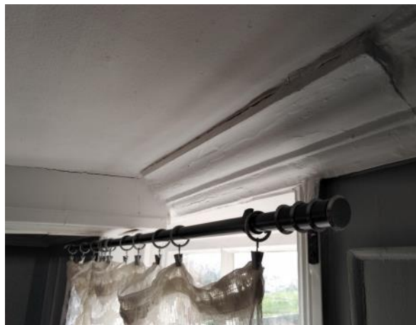
Figure 5.185: Showing how the central ceiling beam sits awkwardly against the western window's architrave.
