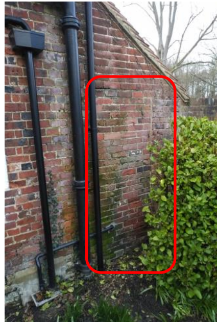
Figure 5.58: Showing the infilled former doorway into the potting shed to the rear of the Breakfast Room.
