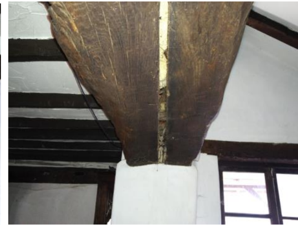
Figure 5.79: Showing the double beam on the opening between the Kitchen and the Breakfast Room. Note the low-grade infill between the beams.
