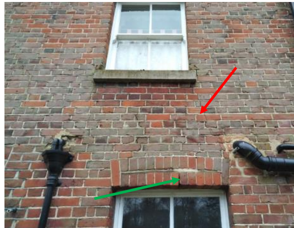
Figure 5.47: Showing the crack from the ground floor central window’s head to the first floor window cill. Also showing the cementitious mortar surrounding many SVPs and overflow pipes.
