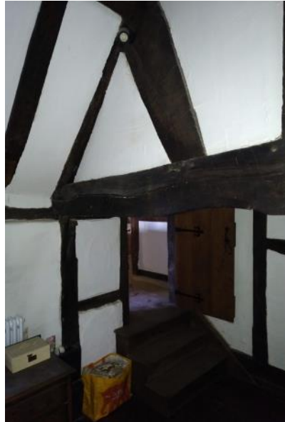
Figure 5.189: Showing the Queen Post truss nearest the entrance doorway into the room and the location of the former brace.
