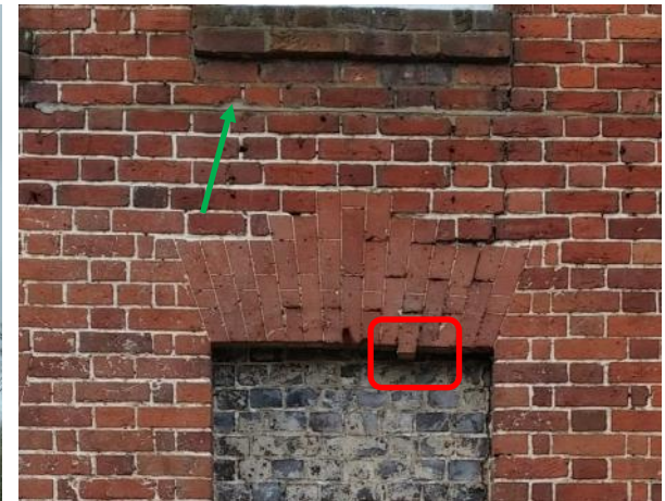
Figure 5.38: Showing the head to the central first floor window to the Front Range's eastern elevation. Note the collapsing brickwork (marked red) and the junction of the previous conservatory (marked green).
