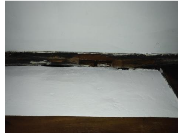
Figure 5.97: Showing the mortise joints for the former posts that once formed part of the wall before the existing doorway between the Snooker Room and Sitting Room was formed.
