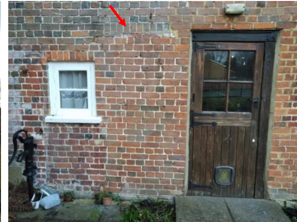
Figure 5.55: Showing the head to the former doorway (marked in red) on the eastern elevation.
