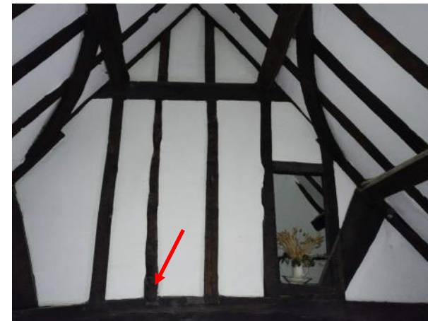
Figure 5.190: Showing the smoking bay doorway (on the right hand side) on the southern end of the Master Bedroom. The loose post is marked in red.
