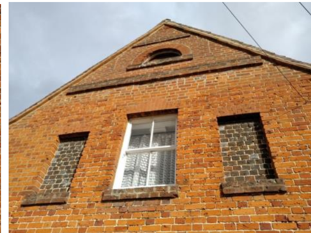
Figure 5.34: Showing the first floor and gable end of the Front Range's western elevation.
