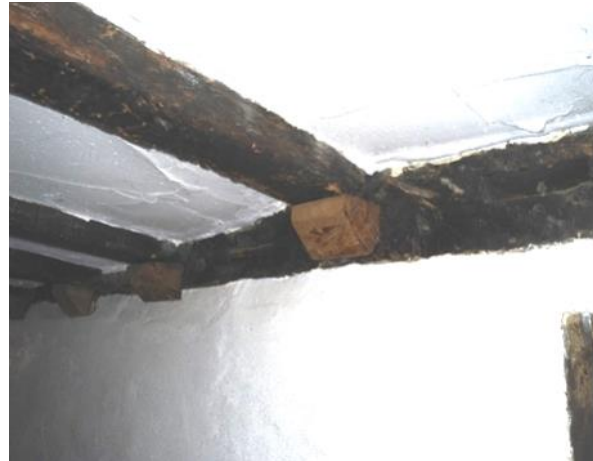
Figure 5.88: Showing the temporary supports where the joists meet the northern beam in the Dining Room.
