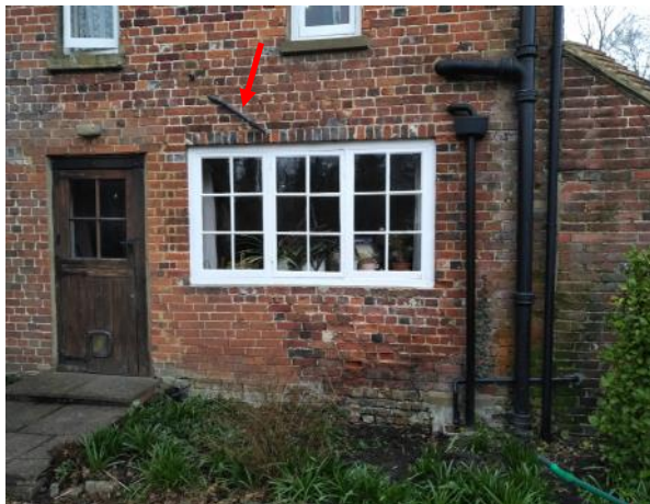
Figure 5.56: Showing the window to the eastern side of the Rear Range. Note the incongruous pipe (marked in red).
