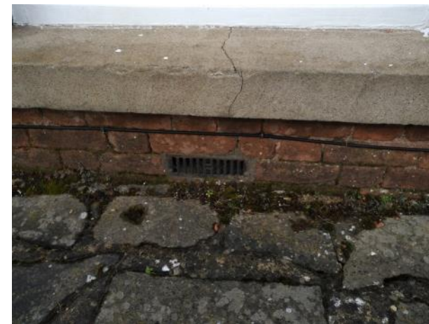
Figure 5.26: Showing the airbrick below the canted bay window. Also note that the concrete cill to the central window is cracked.
