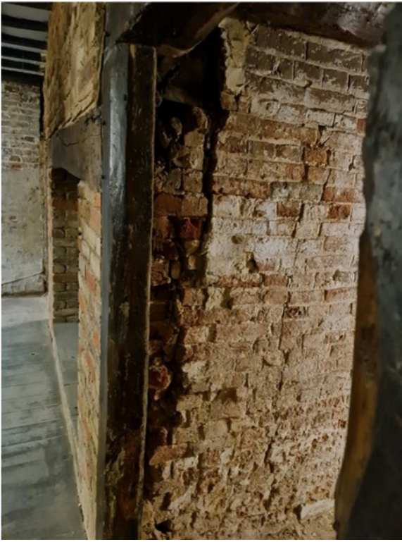
P.7 - GF Lounge - NE Elevation Showing cracked brickwork to chimney Note 7 - DRWG CLT Ltd - P100
