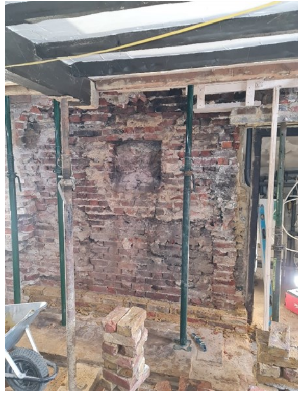
P.6 - GF Kitchen - North Elevation Substandard brickwork removed behind dismantled chimney breast Note 4 - on DRWG CLT Ltd - P100
