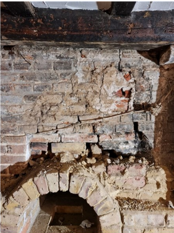
P.9 - GF Lounge - North Elevation Cracked and Substandard brickwork above fake ovens Note 7 - on DRWG CLT Ltd - P100
