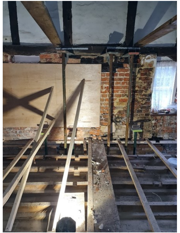
P.39 - 1st Floor En-Suite - North Wall Substandard wall propped to stop collapse Note 20 - on DRWG CLT Ltd - P101
