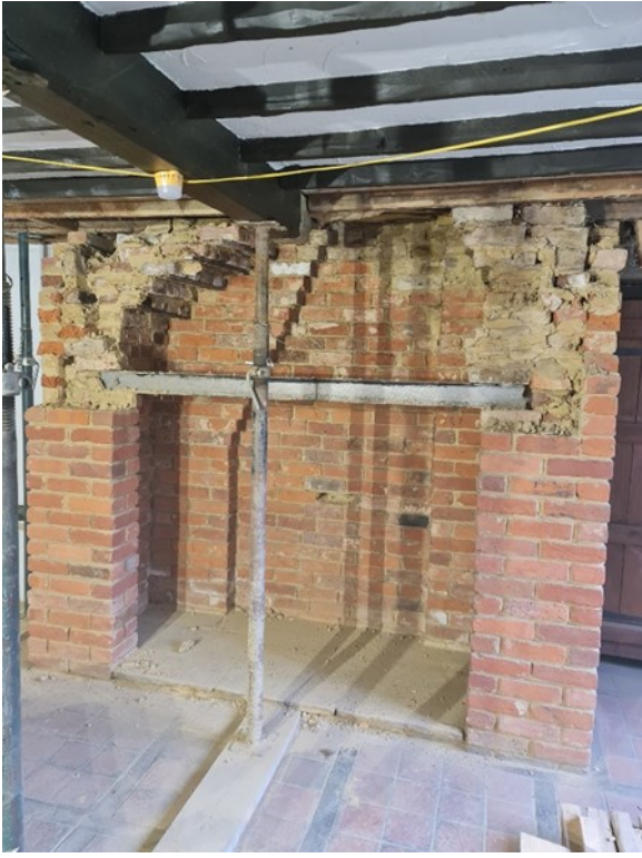
P.5 - GF Kitchen - North Elevation Existing aluminium lintel in fireplace Note 4 - on DRWG CLT Ltd - P100
