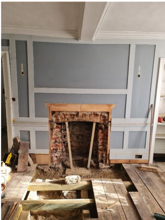
P.32 - GF Music Room - SE Elevation Fireplace showing rotten brickwork
