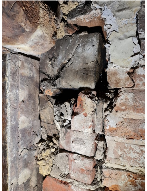
P.8 - GF Lounge - NE Elevation Substandard brickwork to P.7 supporting bressummer beam Note 7 - DRWG CLT Ltd - P100
