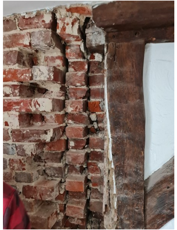
P.51 - 1st Floor Bathroom - NE Elevation Detail showing lack of tie-in
