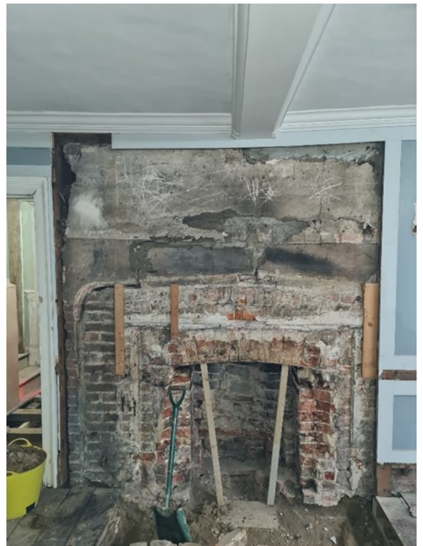
P. 33 - GF Music Room - SE Elevation Fireplace showing additional cracking to supporting arches
