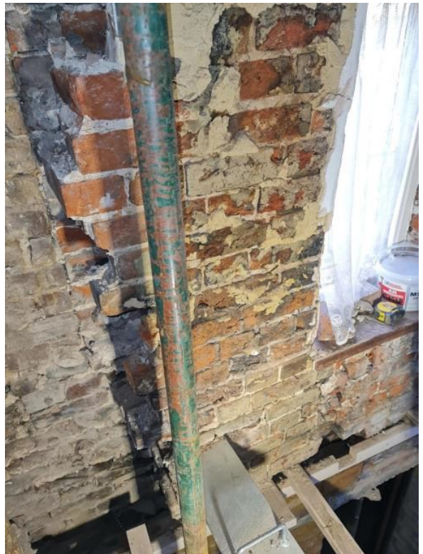
P.41. - 1st Floor En-Suite - North Wall Bad connection between previously altered brickwork Note 20 - on DRWG CLT Ltd - P101
