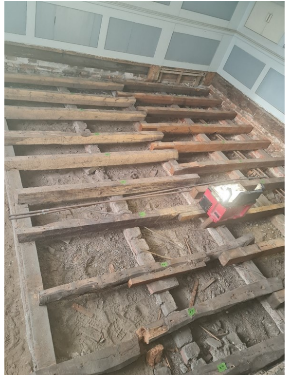
P.31 - GF Music Room - South Elevation Substandard sleeper walls & rotten floor joists
