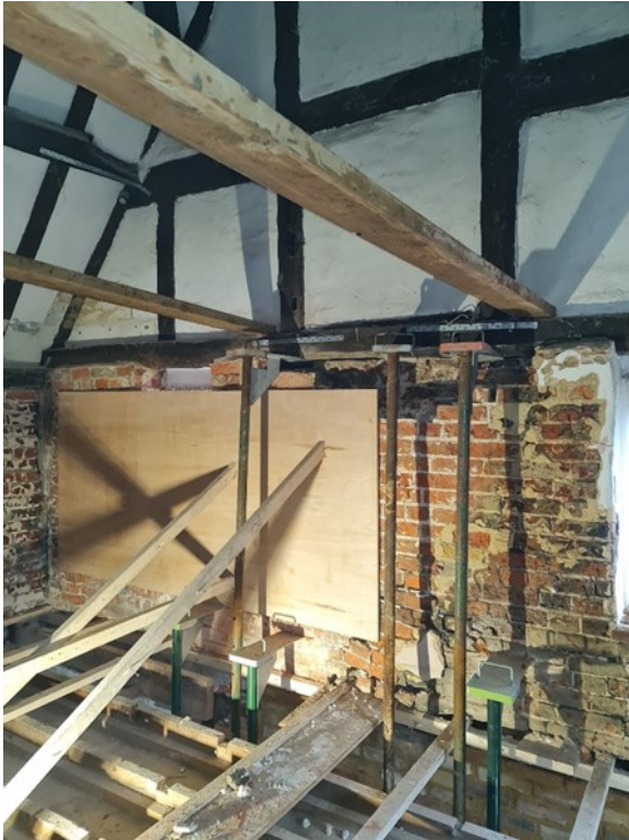
P.40 - 1st Floor En-Suite - North Wall Substandard wall propped to stop collapse Note 20 - on DRWG CLT Ltd - P101
