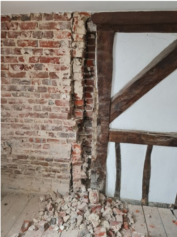
P.52 - 1st Floor Bathroom - NE Elevation Poorly constructed corner return showing unbonded brickwork
