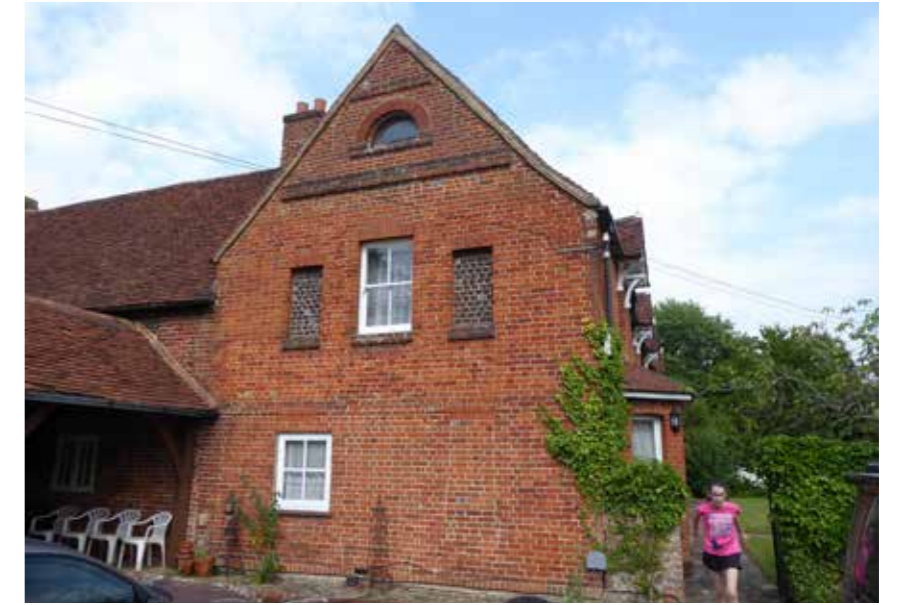
Fig. 24 Evidence of original window openings on West elevation, below brick arched lintels.
