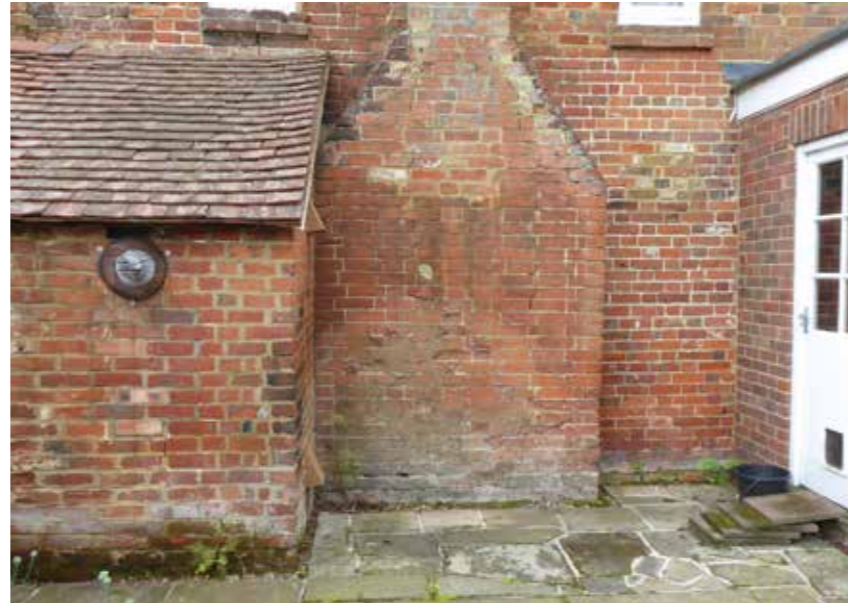
Fig. 20 Multiple areas of damaged brickwork, with poor quality pointing.
