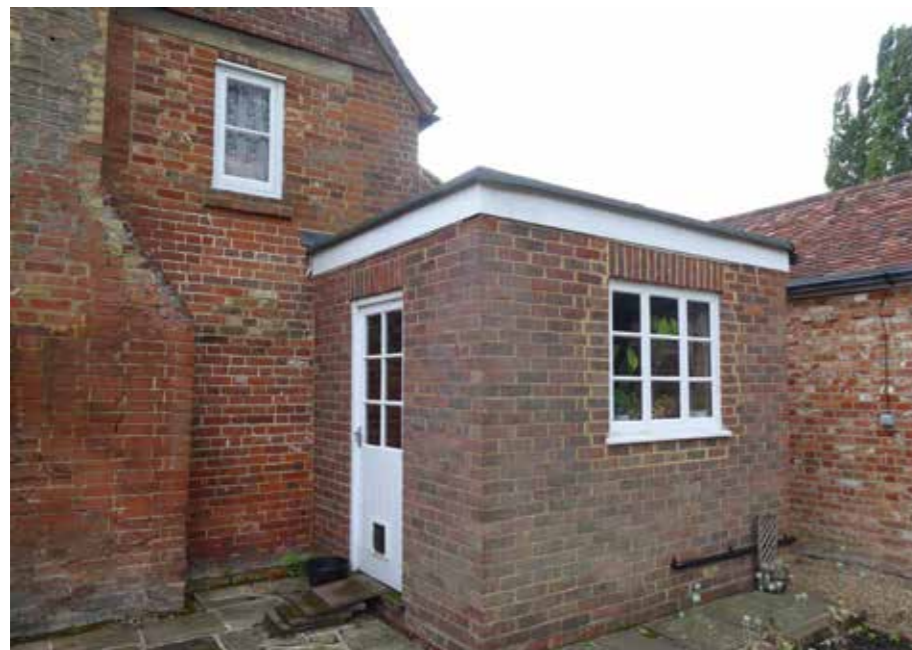
Fig 38: Photo of the existing late-20 th Century flat roofed rear extension, with stretcher course brickwork.
