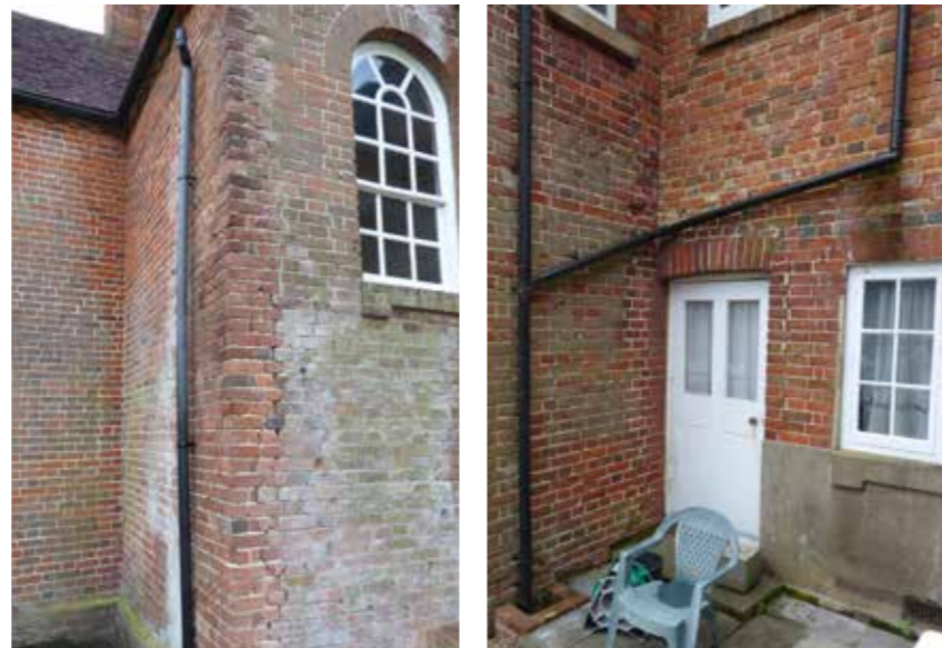
Fig. 21 Evidence of cracks externally in the brickwork.(Refer to S.E. Report for details.)
