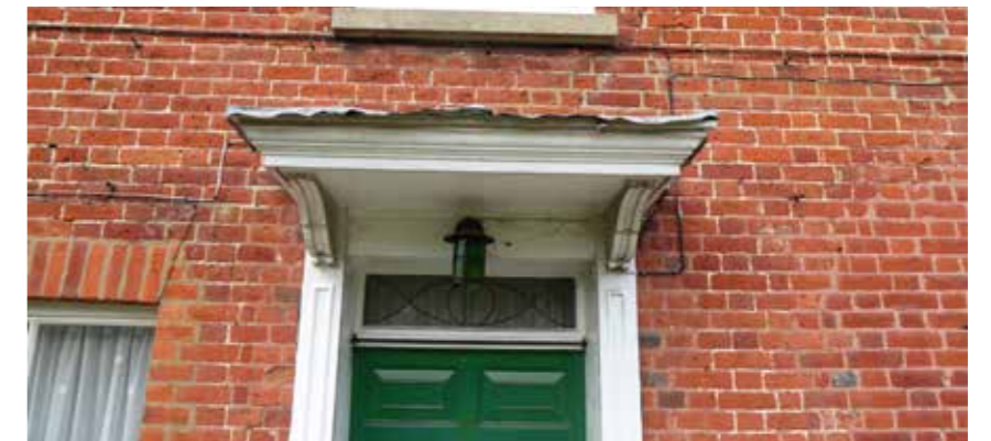
Fig. 26 Existing flat roof canopy with deteriorated lead detailing.
