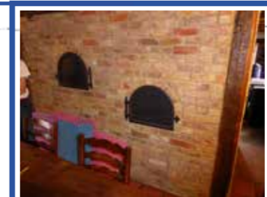
Fig. 10 Unsympathetic alterations to existing inglenook (faux brick ovens).
