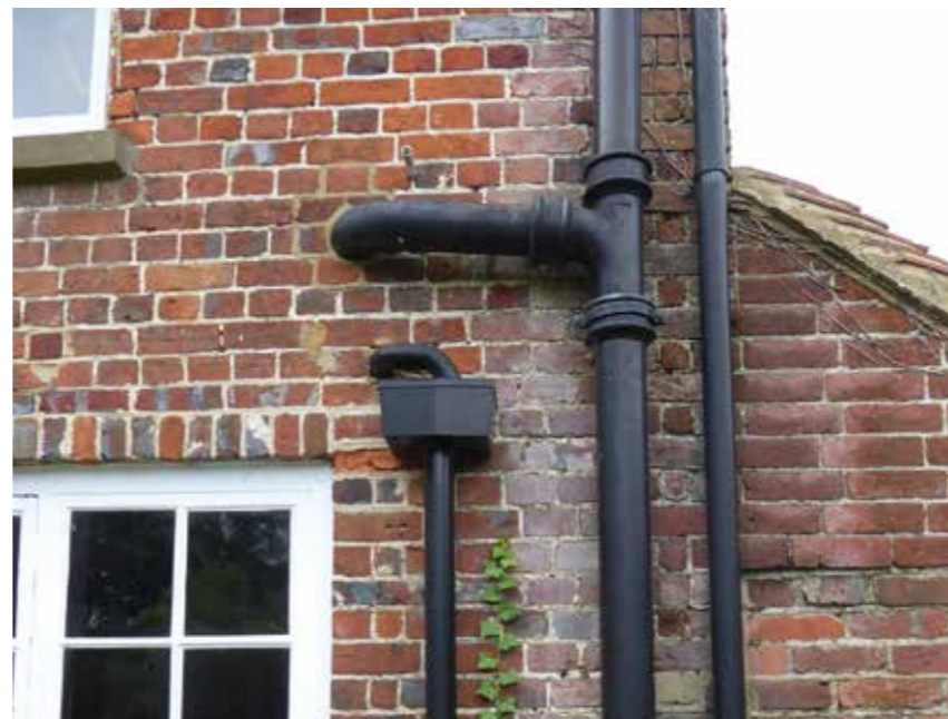
Fig 34: External rainwater goods and soil stacks proposed to be modified and rationalised
