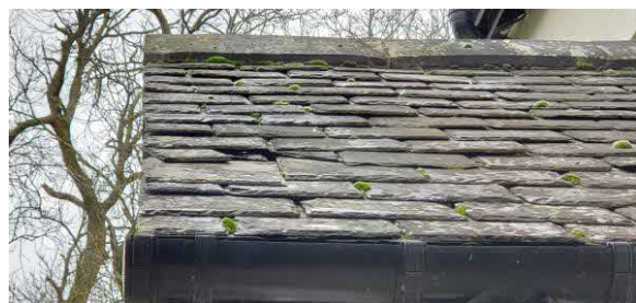
8 Broken tile on porch (not impacted by works)
