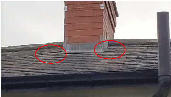
5 Slight raised slates by chimney
