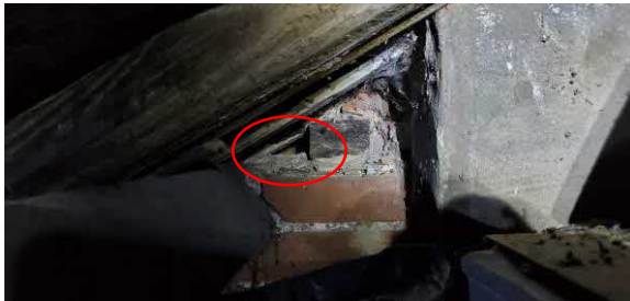
11 Wall dividing the two roof voids (gap highlighted)
