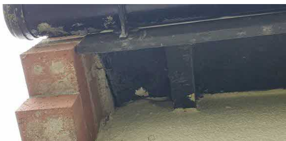
7 Gap at soffit of mono-pitched roof (scoped out as bat roost)
