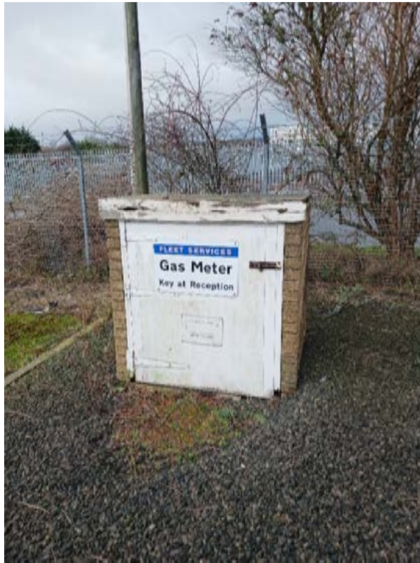
Photograph 7 – Gas meter adjacent to western boundary. Photo taken facing W.
