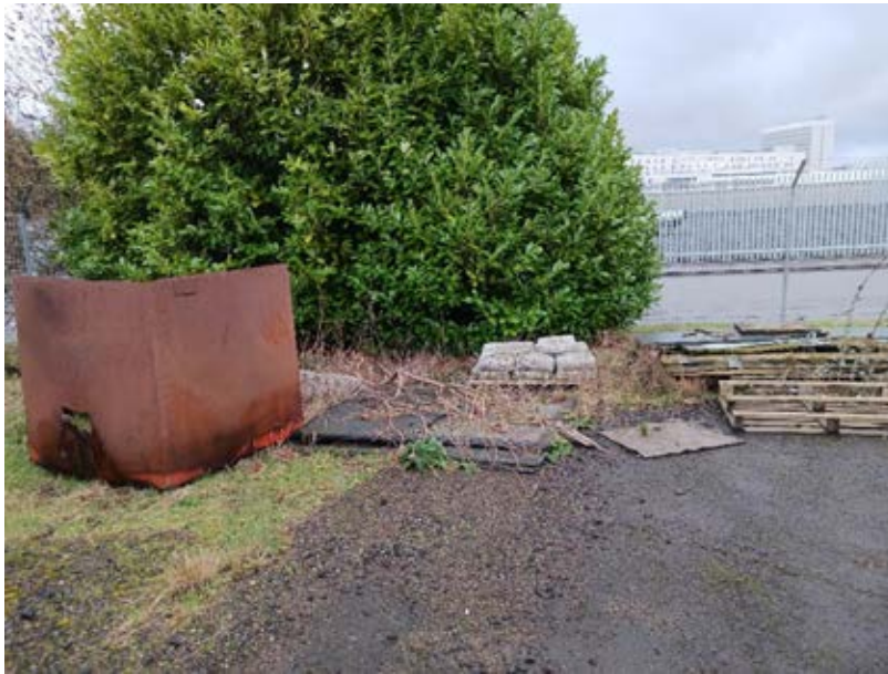
Photograph 9 – Leftover materials: bags of cement, pallets, metal and plastic sheeting. Photo taken in south of site, facing W.
