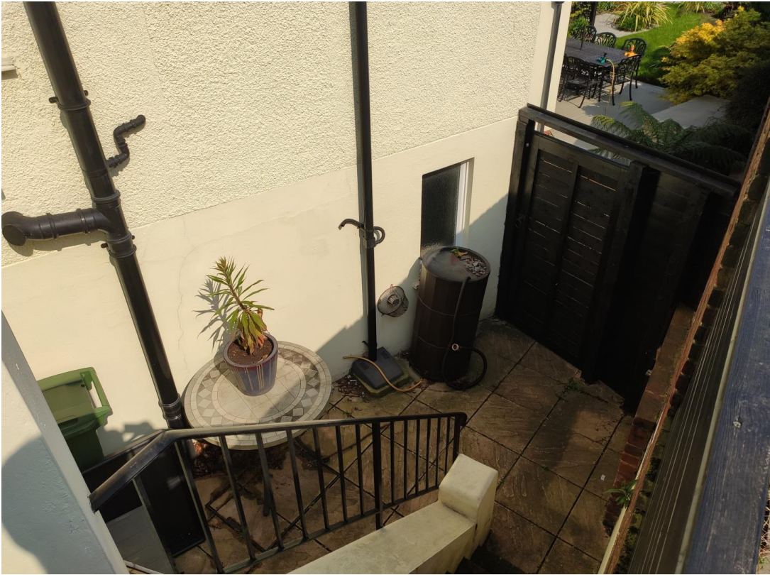
Figure 5: Photo of southern side of property showing the lower ground floor area
