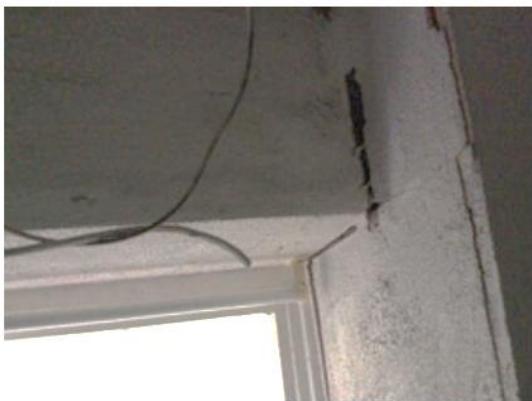
Picture 1: Internal cracking to WC
