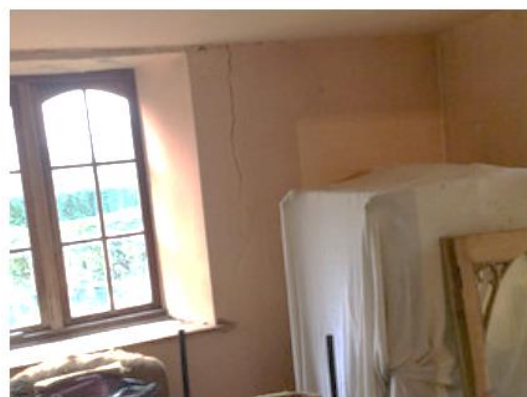
Picture 2: Internal cracking to Left Hand room
