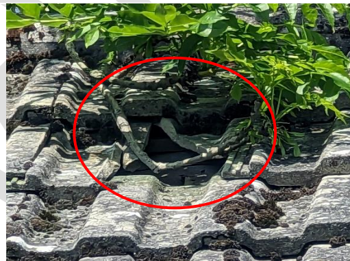
Figure 4.11. Broken tiles on the southeastern elevation of the bungalow
