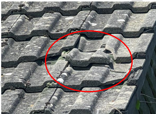
Figure 4.10 Broken tile on the southeastern elevation of the bungalow
