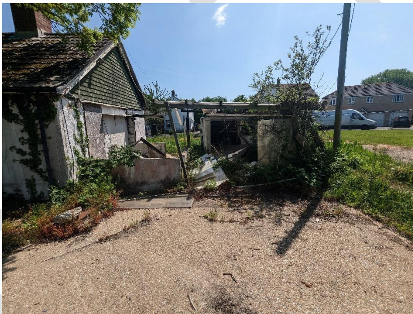
Figure 4.7. Burnt down garage at the southern extent
