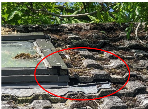
Figure 4.12. Gap under the flashing of the skylight on the southeastern elevation
