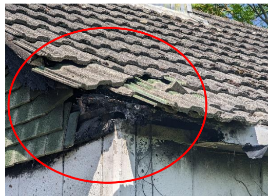
Figure 4.13. Gap within the damaged soffit on the southern corner of the dwelling
