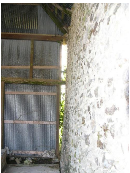
Wall lean out
