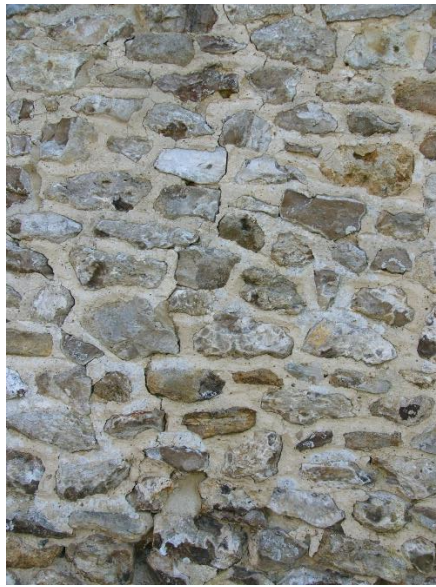
Mid wall movements crack
