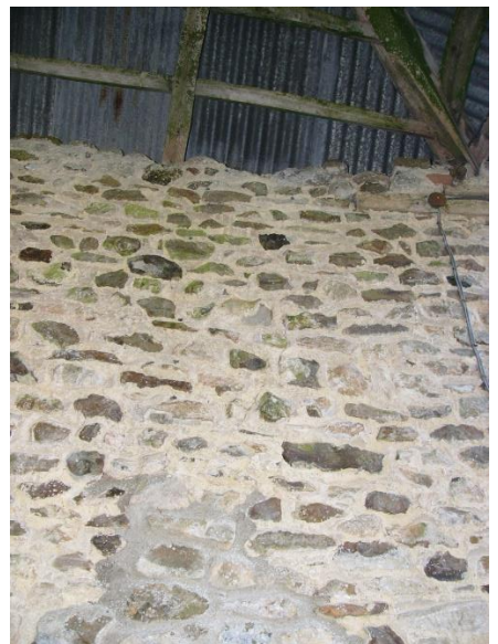
Wall crack and truss bearings.
