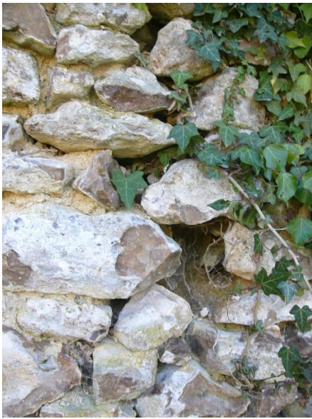
Wash out at base
