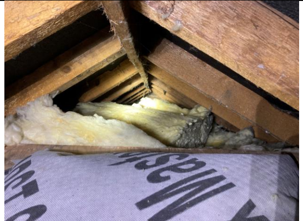
Photo 4 Small void above main roof
