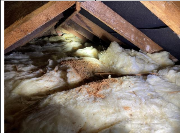
Photo 5 Small void above main roof
