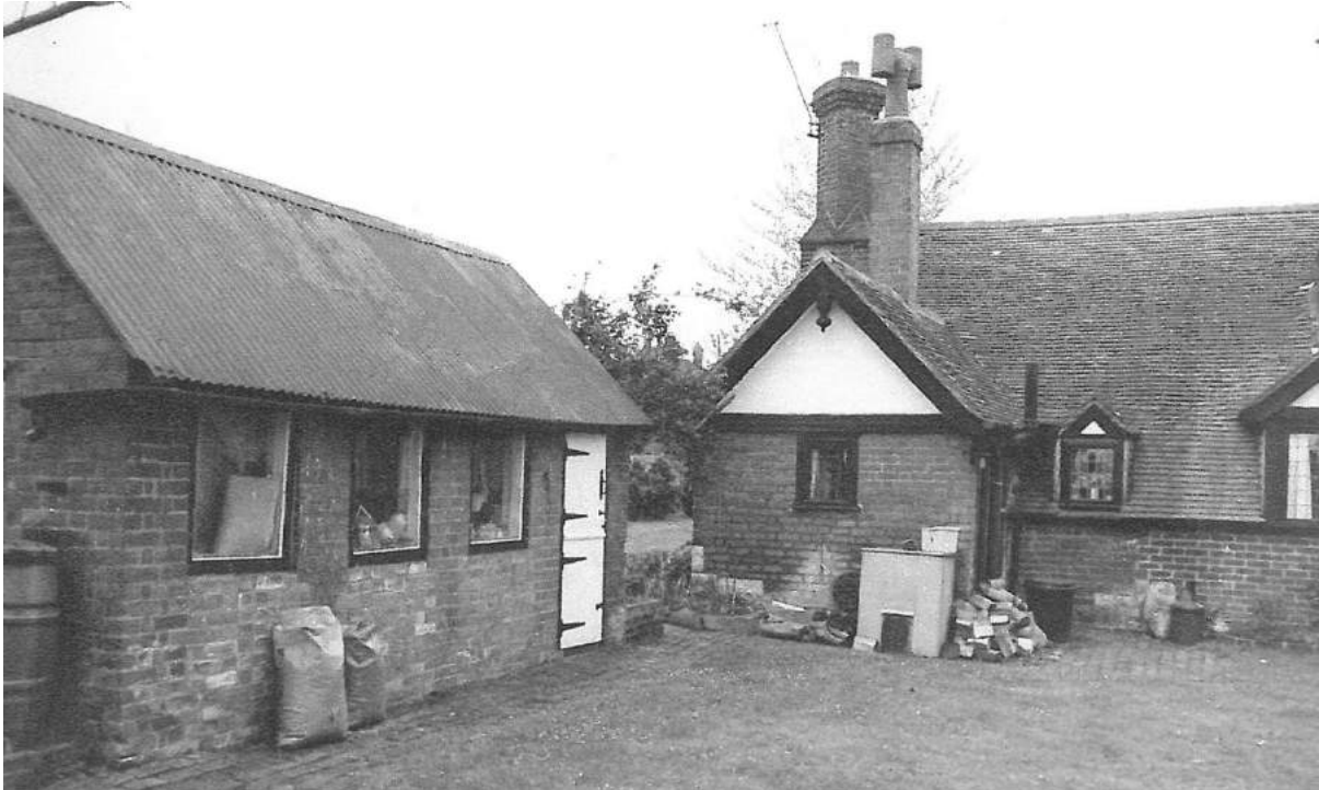
Above: Photograph of rear elevation c1986, clearly visible is the original rear extension and brick outbuilding. Brickwork beneath the two rear dormers demonstrates infill of an originally open air space.
