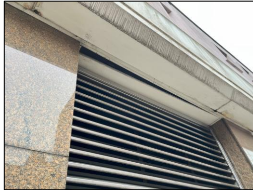
Photo 2: Gap behind a dislodged wooden board approx. 2.5m from the ground, above one of the shutters
