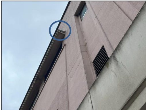
Photo 3: Loose roofing felt covering a window ledge on the 2 nd storey
