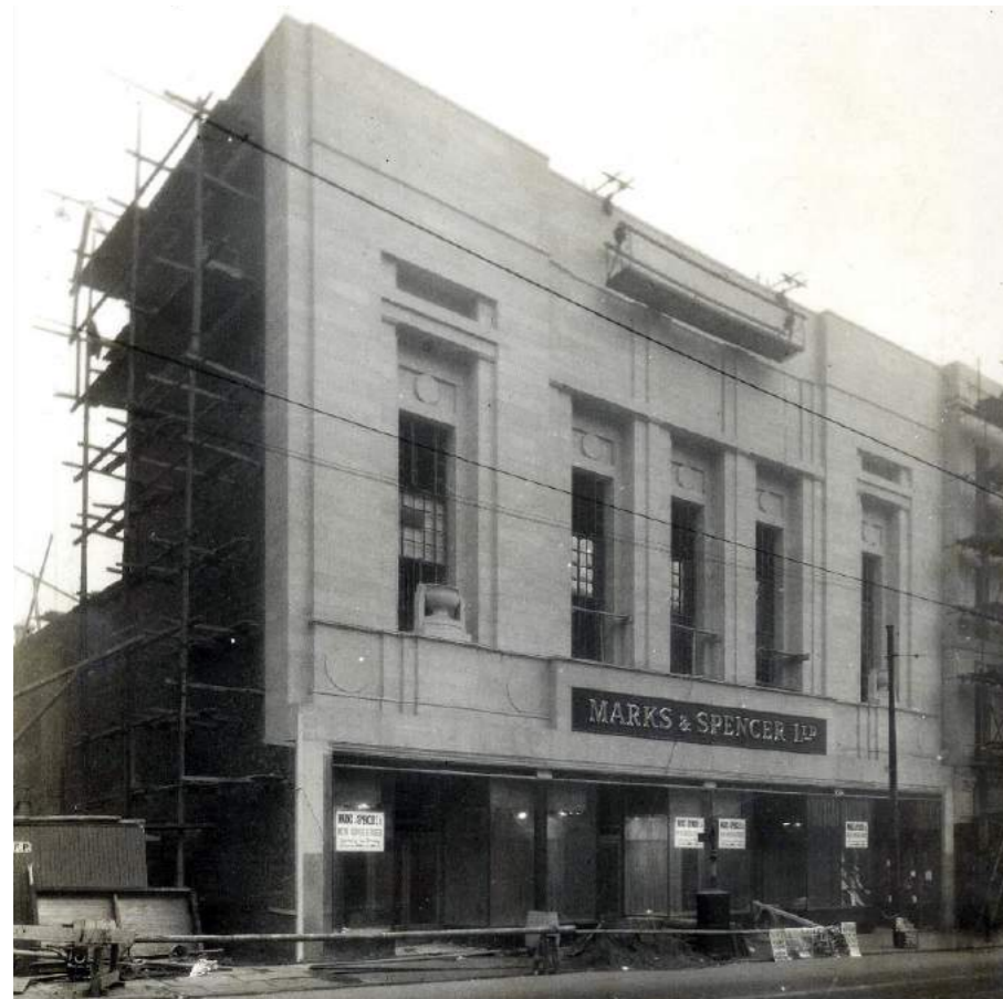
The original facade under construction - the modular design is poorly related to the floors that sit behind it.
