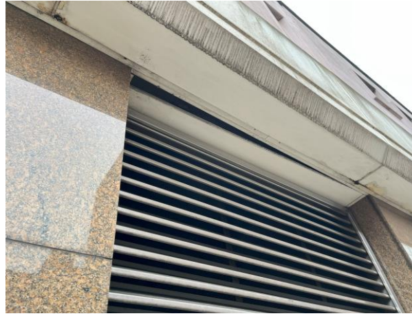
Photo 2: PRF- gap above the shutter, in the northern aspect.
