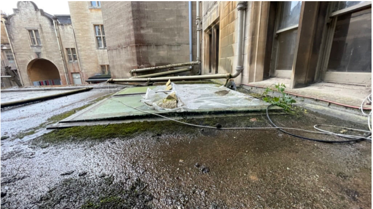
08 Looking east towards rooflights r102 and r102. Concrete substrates to minimal falls with asphalt roof covering and solar reflective paint finish, now all in need of replacement. Moss growth is visible where roof retaining water immediately adjacent to rooflight. Roof falls to just 2no outfalls to south west corner of courtyard (rw01) and at north end of roof (rw02) – see roof plan drawing 139/100 for details.
