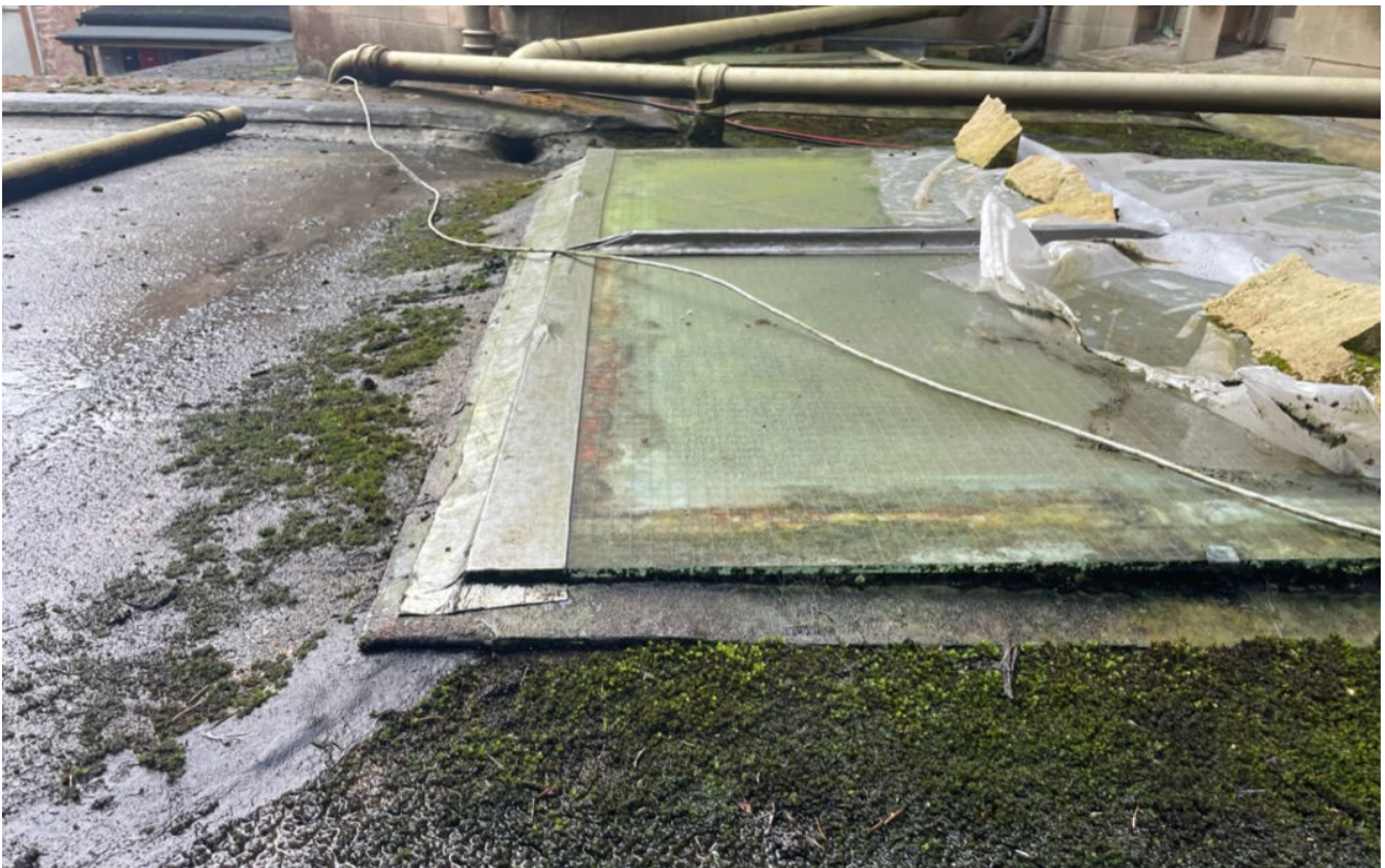
06 Rooflight r102 looking east. Edge detail is leading to repeated water ingress due to of lack of adequate vertical upstand, especially in storm conditions. Note minimal 40Ø of roof outlet (rw01) which leads to surcharging in storm conditions.
