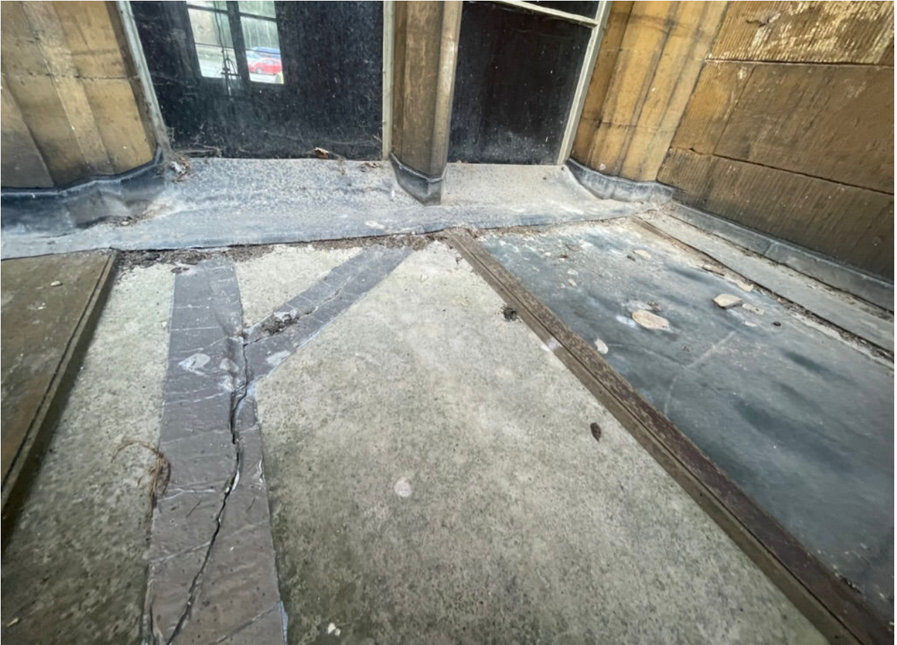
12 Looking west to end rooflight r105. Replacement design similar to r104 with one glazing panel replaced with [damaged] asbestos cement sheet sealed with flashband. Northern edge of rooflight is flashed into adjacent ashlar walling.
