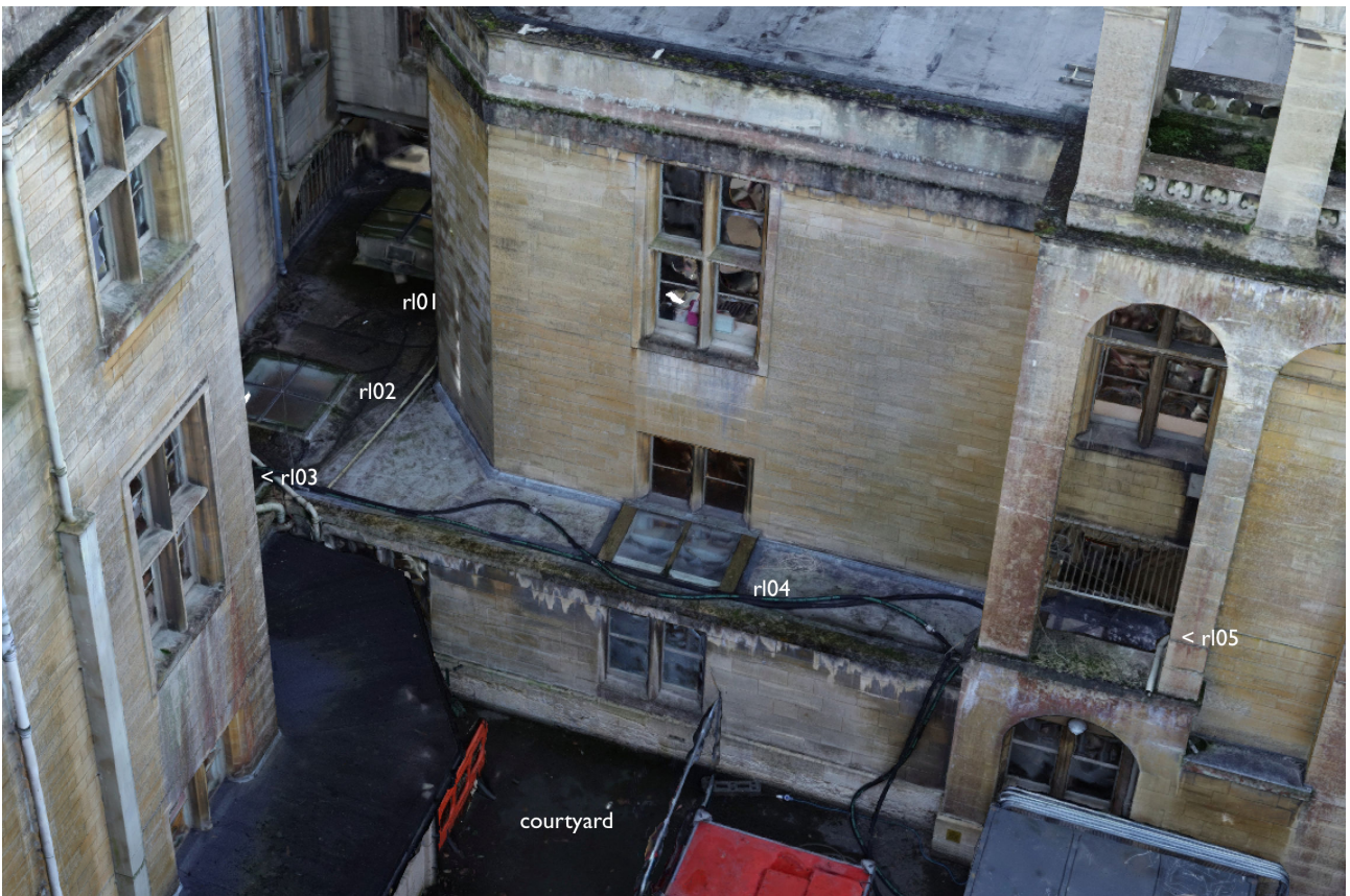
02 South west corner of north east courtyard with Belvedere tower visible to right of the image. Single storey flat roof to minimal falls with intermediate rooflights to corridor and service areas at lower ground floor level.
