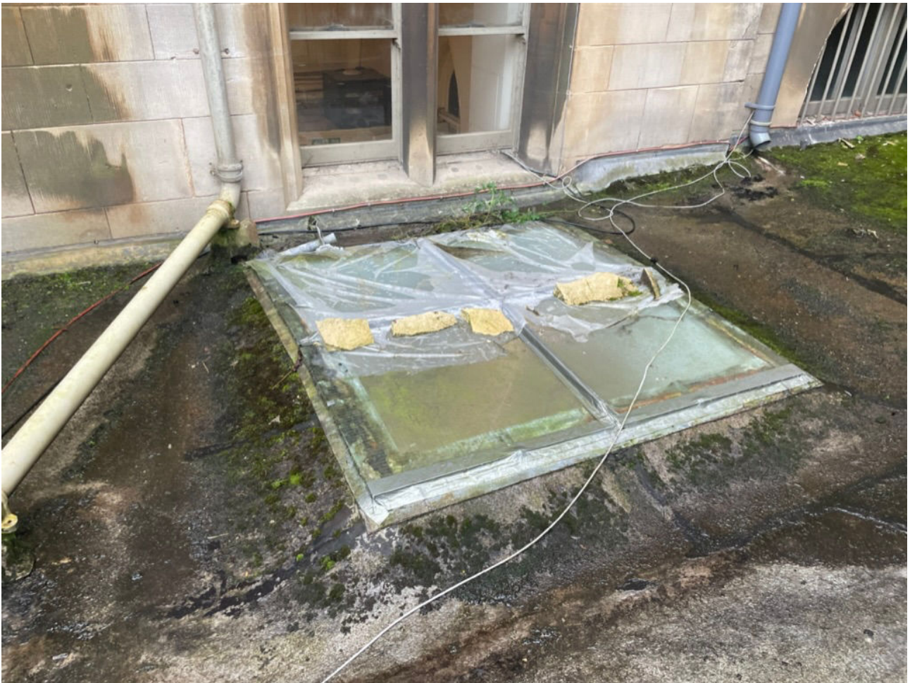
05 Rooflight r102 looking south towards wn02. Modern Georgian wired glass with inverted T section iron beams, patched with flashband and more recently subject to emergency protection with polythene sheet to resist ongoing water ingress.
