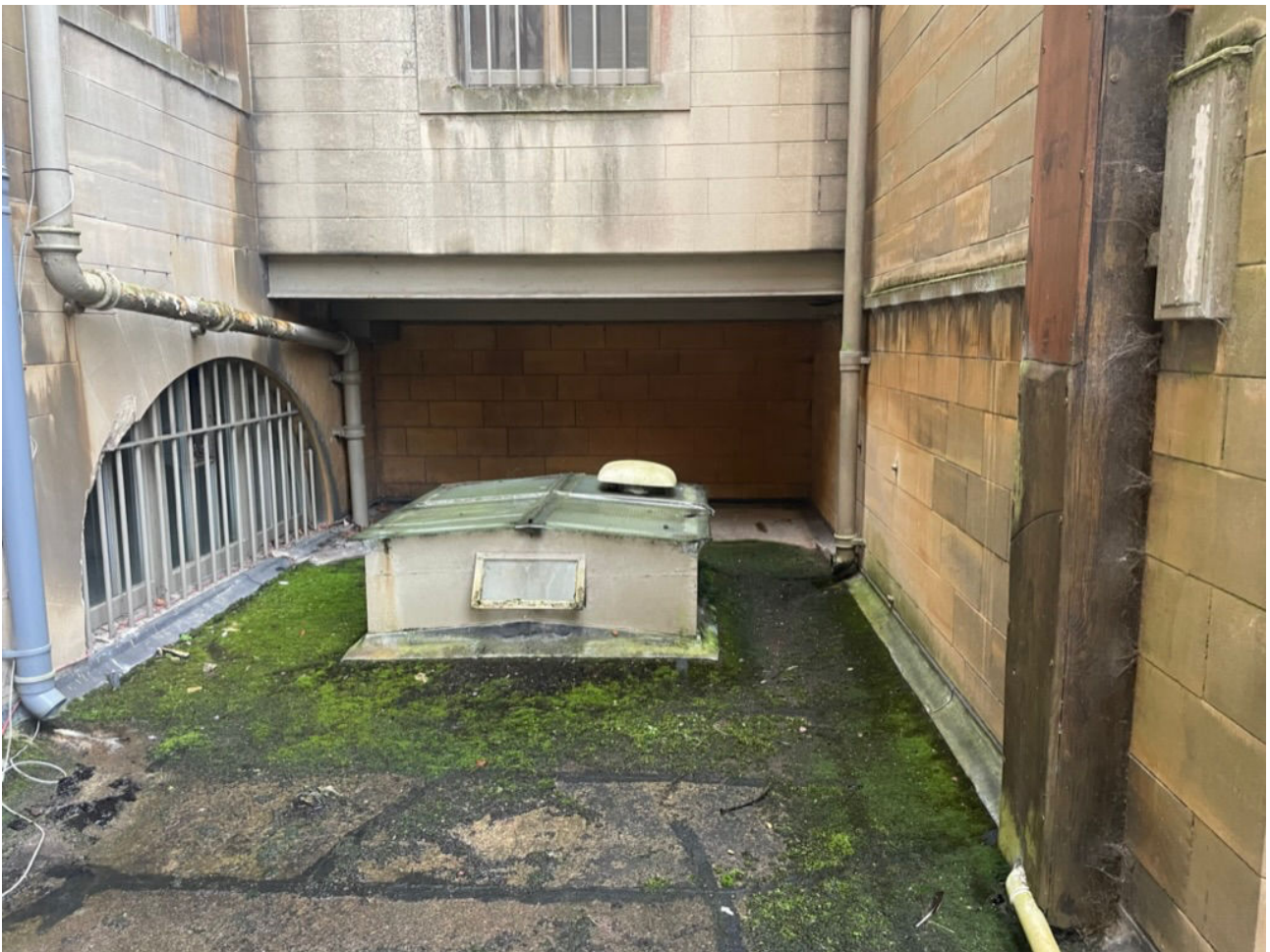
04 View of rooflight r101 looking west. Replacement Georgian wired glass rooflight with inverted T section iron beams. Much patched with flashband over leaking lead capped joints (itself a remedial detail attempting to improve on the original linseed oil putty weathered joints to glazing bars).
