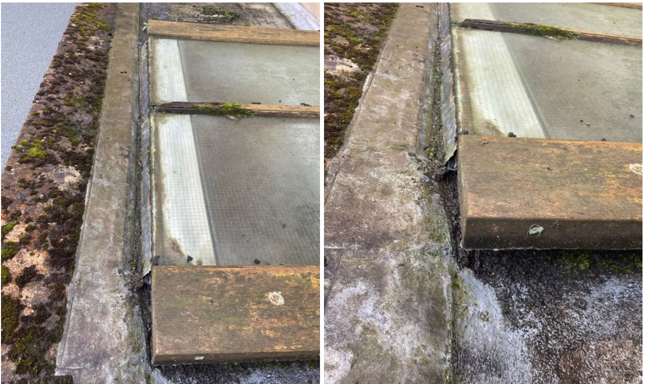
10-11 Looking north to rooflight r104. Narrow gutter to edge of r104 silts up and due to minimal upstands resulting in regular water penetration internally. Note also decaying moss covered glazing bar in need of replacement.
