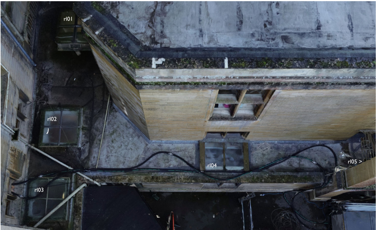
03 Aerial view of south west corner of north east courtyard highlighting location of concealed rooflights in slot between principal range and north east service court.
