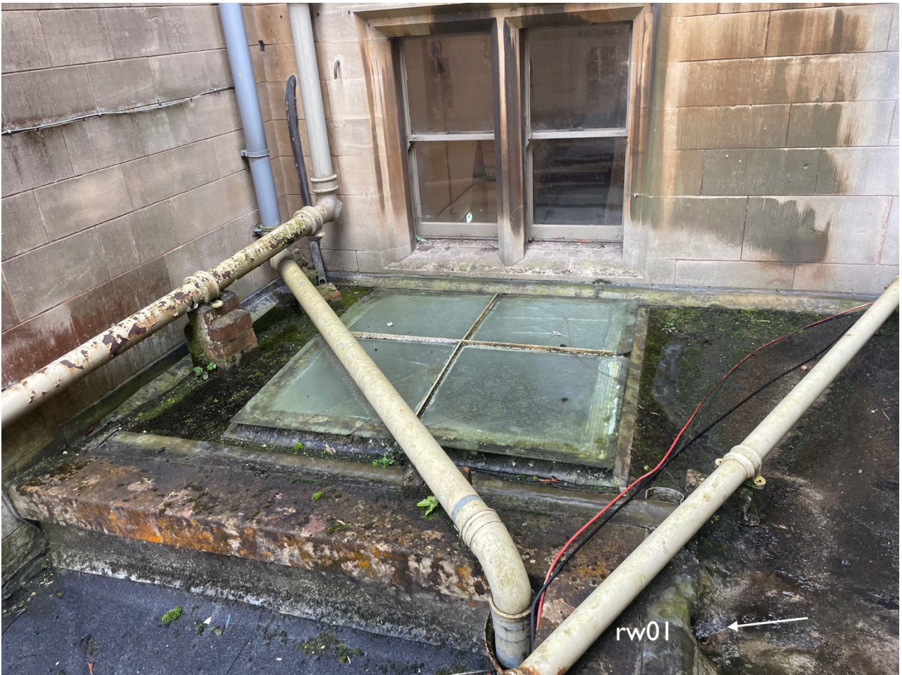
07 Rooflight r103 looking south towards wn01. Repeat of poorly designed perimeter upstand as r102, which replicates all the defects associated with intermittent water ingress. Note roof outlet (rw01) which tapers to 40ø passing through wall before discharging to hopper beyond coping.
