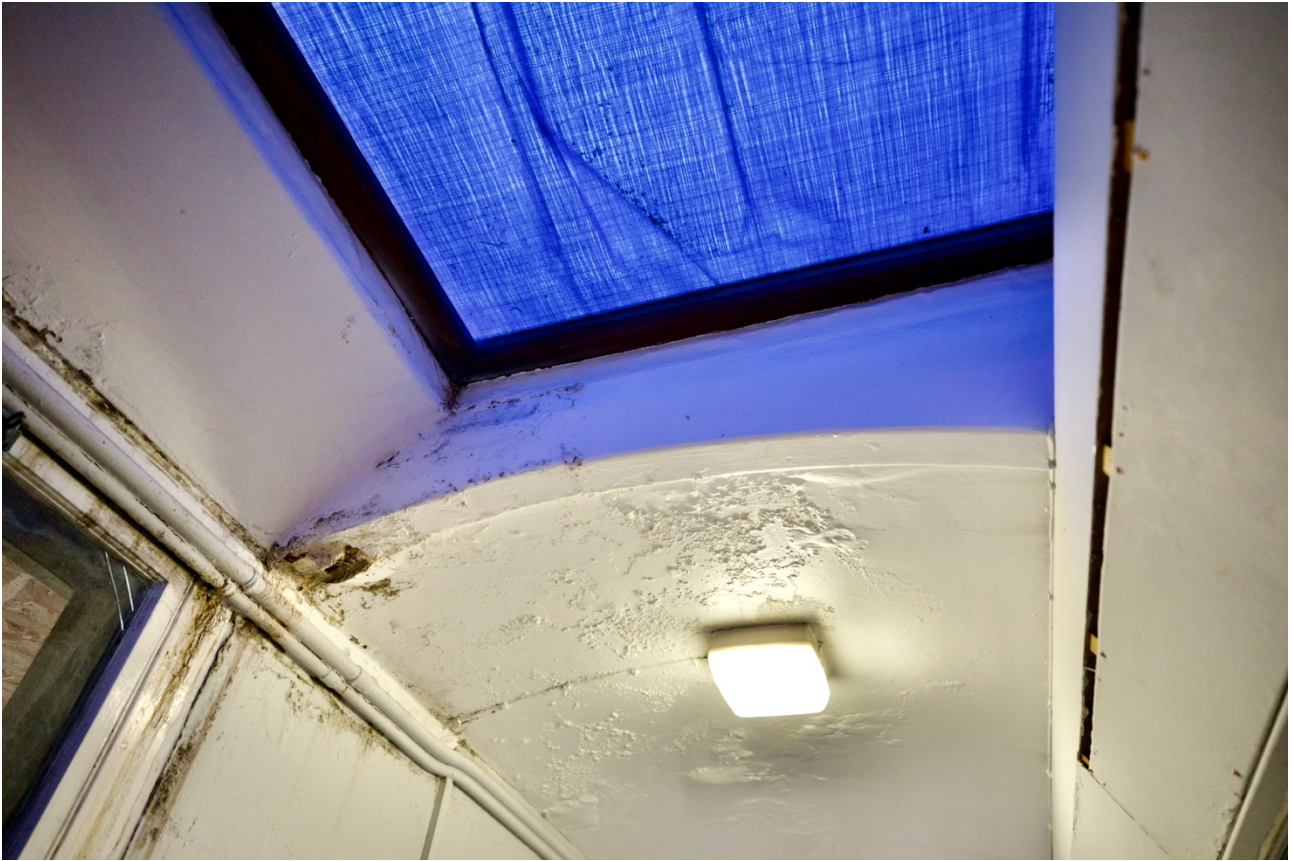
23 Detail of r104 looking south. Water penetration and algal/mould growth to south west corner of rooflight.
