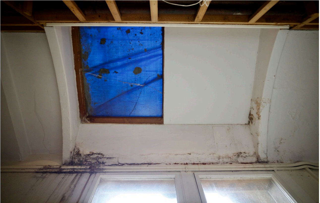
26 Looking east below r105. With significant repeated water penetration to trimmed reveals. Right hand side of rooflight has been boarded-in internally with plywood and asbestos cement board externally – see 12-14. Main source of water penetration to north east corner of rooflight is constrained (and debris filled) narrow gutter to roof outlet.
