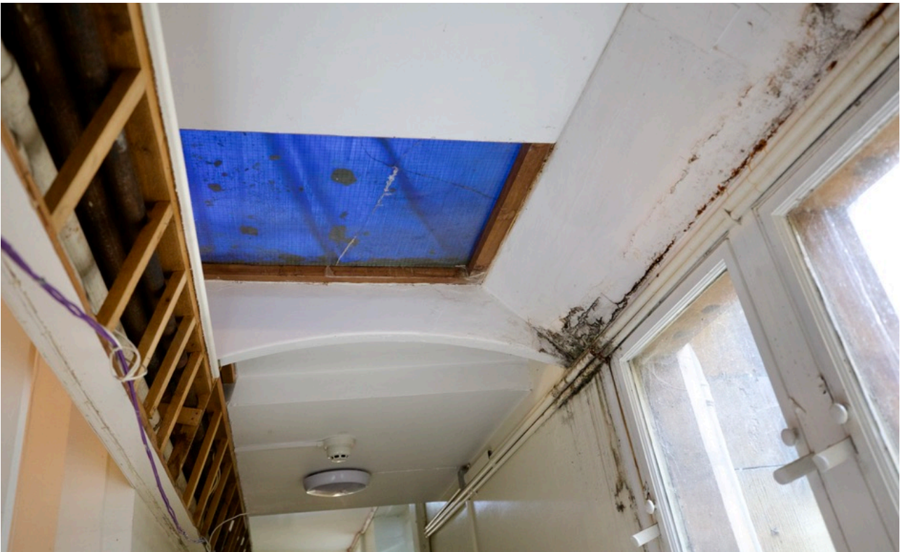
27 Looking north below r105. Mould growth to right hand corner of rooflight corresponds with adjacent 40ø roof outfall to downpipe to external face of wall. Proposal to introduce new rooflight with narrower perimeter kerb will allow install of wider gutter and enlarge core drilled outfall through wall (that is capable of maintenance to mitigate build-up of silt).
