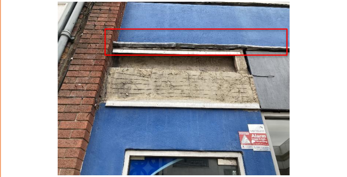
PLATE 3 SHOWING MISSING CLADDING AND LIFTED FLASHING (F1)
