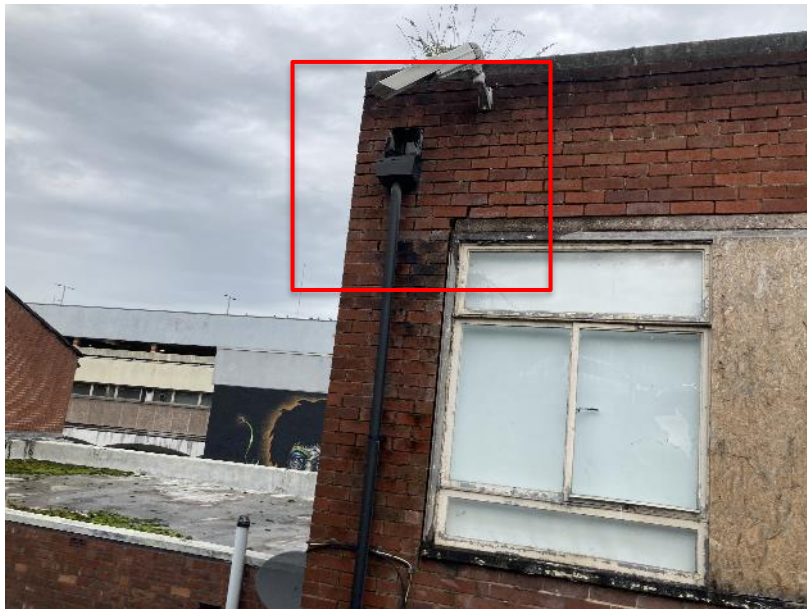
PLATE 5 SHOWING CREVICES SURROUNDING PIPEWORK AND WINDOW (F2)
