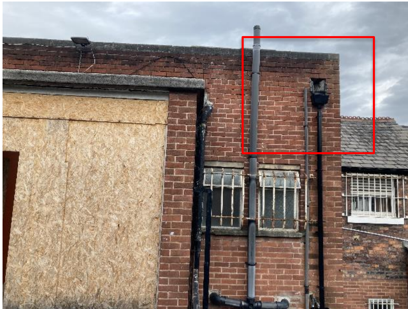
PLATE 6 SHOWING GAPS SURROUNDING PIPEWORK (F3)
