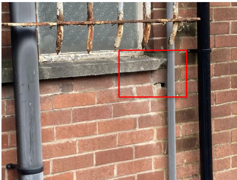
PLATE 7 SHOWING DAMAGED BRICKWORK (F4)
