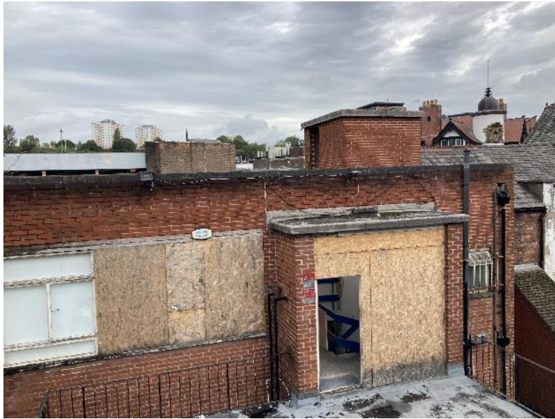
PLATE 4 SHOWING DAMAGED SOUTHERN ASPECT
