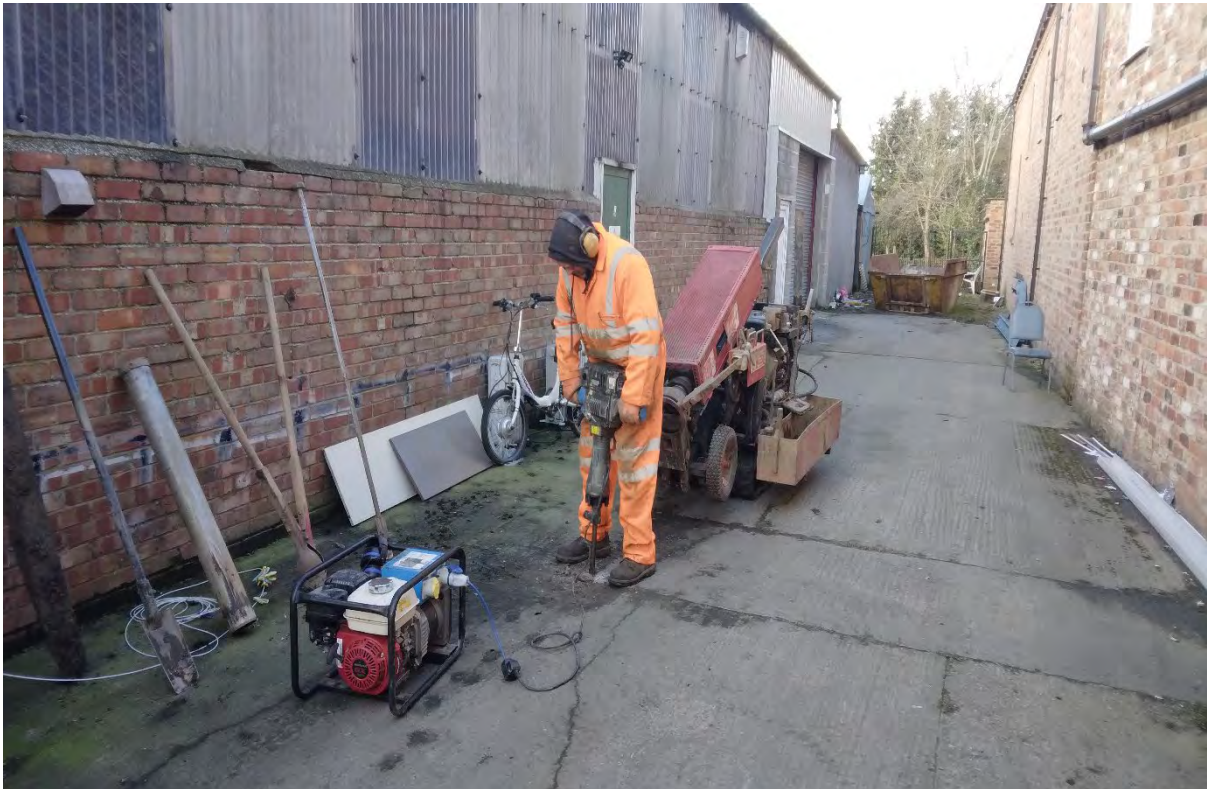
View northwest through the site towards BH04 during initial breaking out of Hardstanding.
