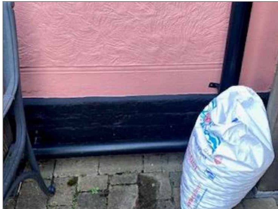
BRICKWORK PLINTH BELOW RENDER TO BE PAINTED MATT BLACK TO MATCH EXISTING
