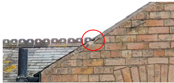
4 Gap in mortar
