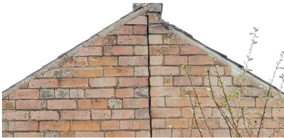
3 Gap between neighbour's extension
