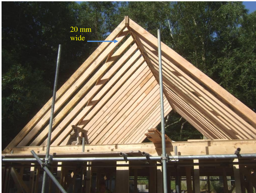
Figure 3- Photographic example of the double ridgeboard detail installed within the 'Bat Barn' and example of the open flight area under the roof covering required between the roof frames and gables internally
