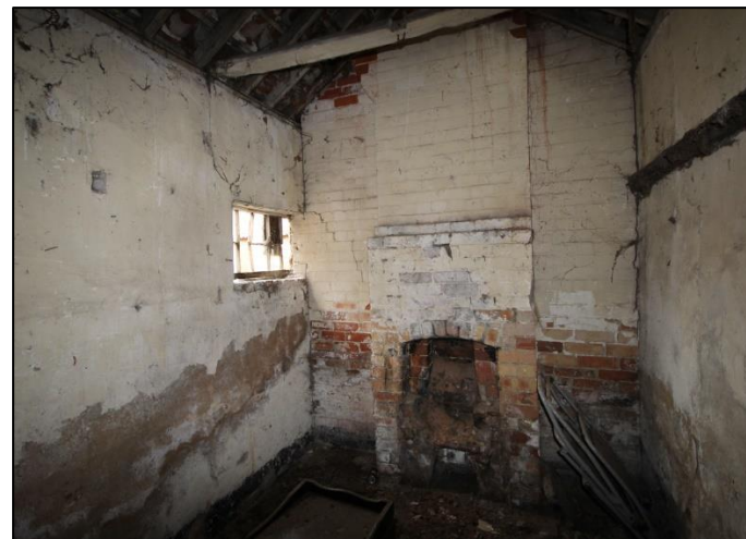
Plate 20: Internal view of western wing of Building A looking south (northern room).
