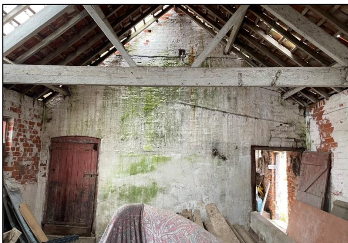
Plate 43: Internal view of Building C looking south, with party wall to Building D.
