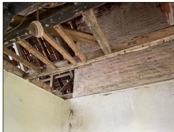
Plate 41: Internal view of roof structure and two-third height lime-plastered walls to abutting room.
