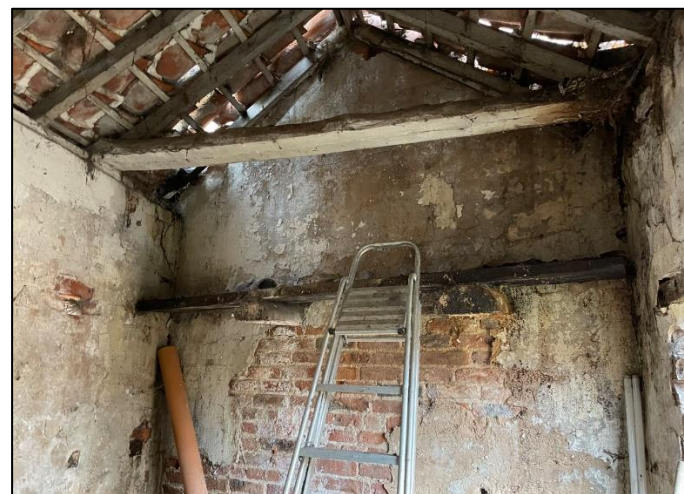
Plate 21: Internal view of western wing of Building A looking north (northern room).
