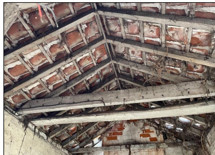
Plate 23: Internal view of roof to western wing of Building A looking north (southern room).
