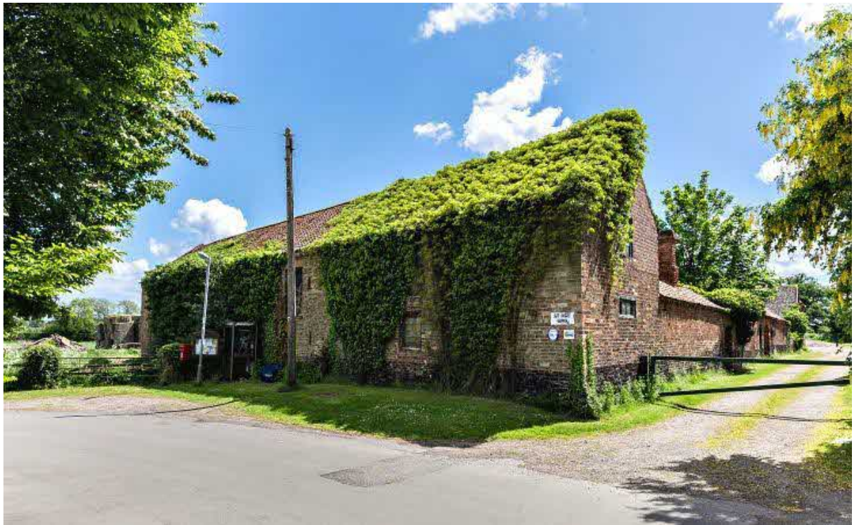
Photograph 1: Building A and Building B taken from the north-west, showing the two-storey height and the climbing plant covering parts of the roof.
