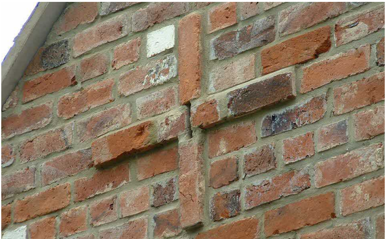
Figure 3: an example of the access slit to be installed within the eastern gable.
