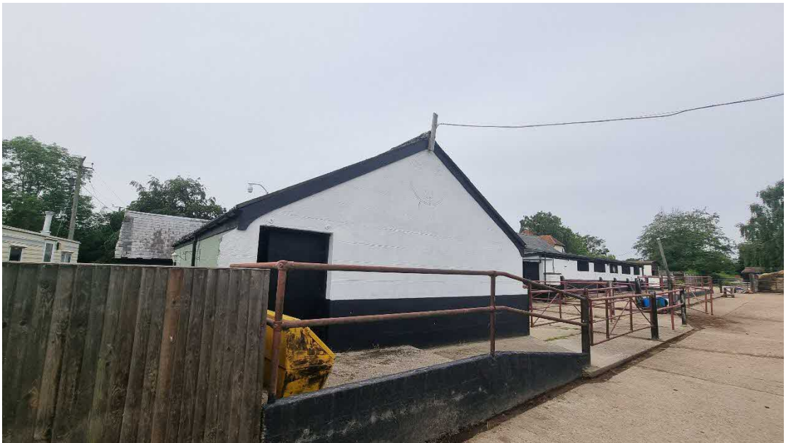
Fig.8: North elevation of the milking parlour with the listed farmhouse concealed by the stables and historic barns to the right.
