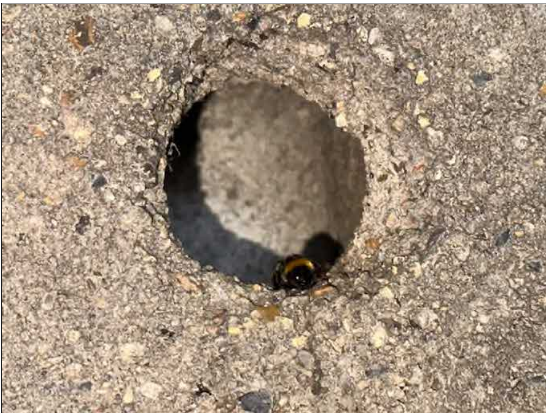
h) Bumble bee in cavity wall on northern aspect.
