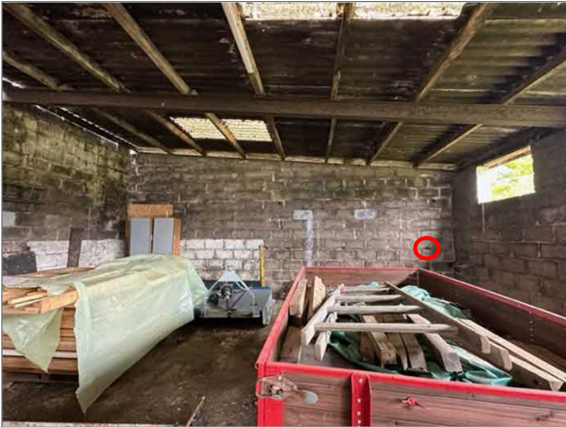
e) Building 3: Northern aspect, internal. The gap circled was inspected with an endoscope.
