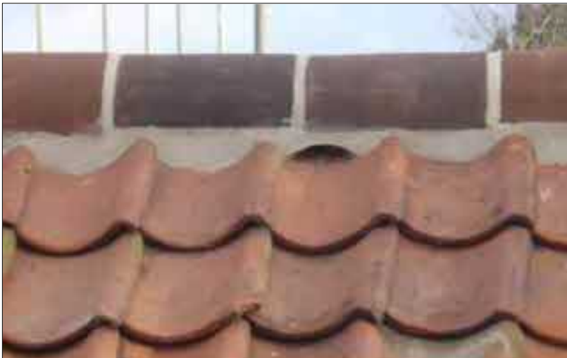
b) Gap beneath ridge tile of reclaimed clay pantile roof
