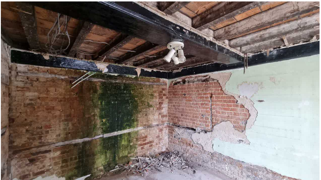
Fig.12: Water ingress from damaged chimney stack and modern gypsum plaster to opposite wall which has blown.
