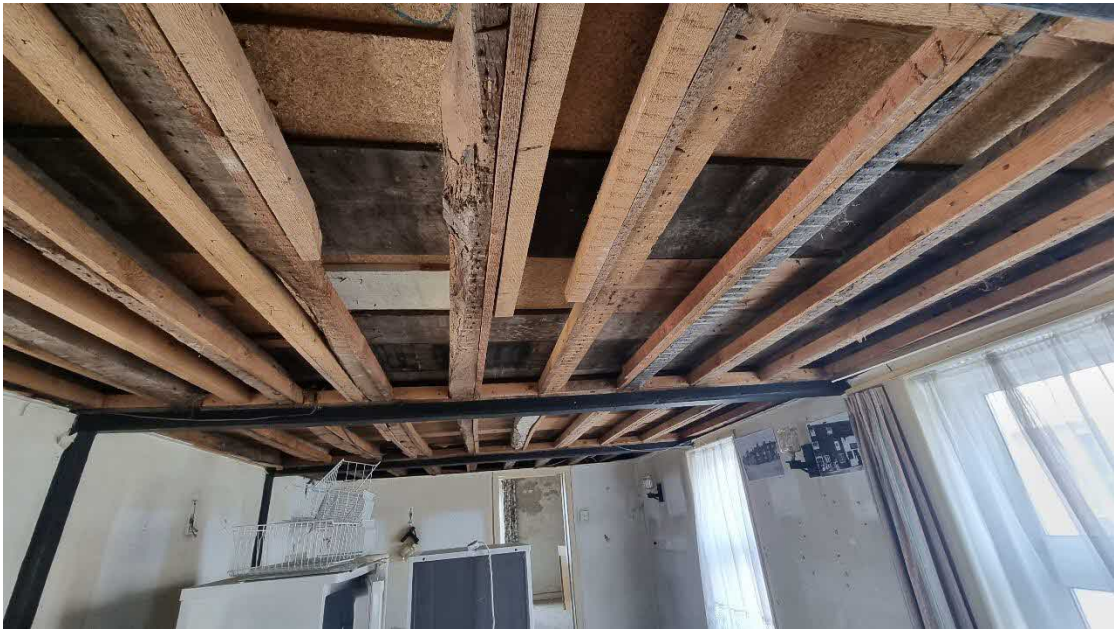
Fig.11: The addition of modern timbers to in situ joists appear have been inserted to strengthen the floor.
