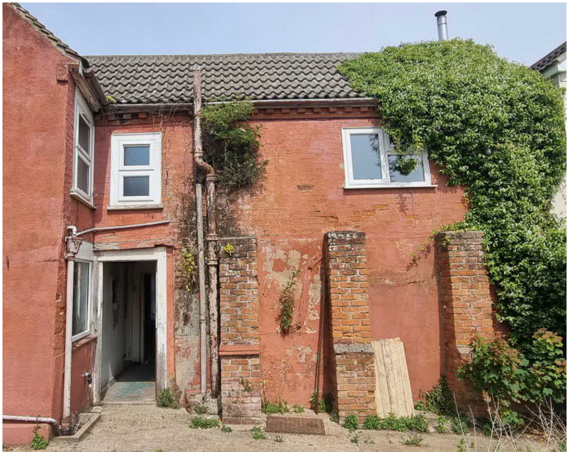
Fig.7: Buttresses and parrass plate to southeast elevation. A previous intervention to resist the walls movement. Also of note is the location of the door were the southeast elevation meets the northeast elevation which has a window perpendicular to the doorway. This is not a suitable location for this opening as it results in a little of no lateral support for the main southeast elevation. (See para 4.4.1 of Steven Heard Associates structural report).
