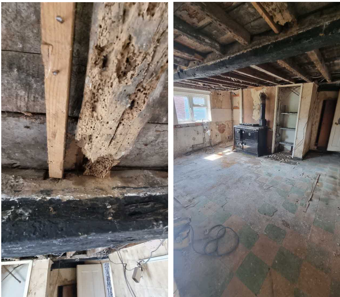
Fig.10: Example of floor joists which have historic and archaeological value and show signs of irreversible decay. The planning system allows for their removal without planning permission.
