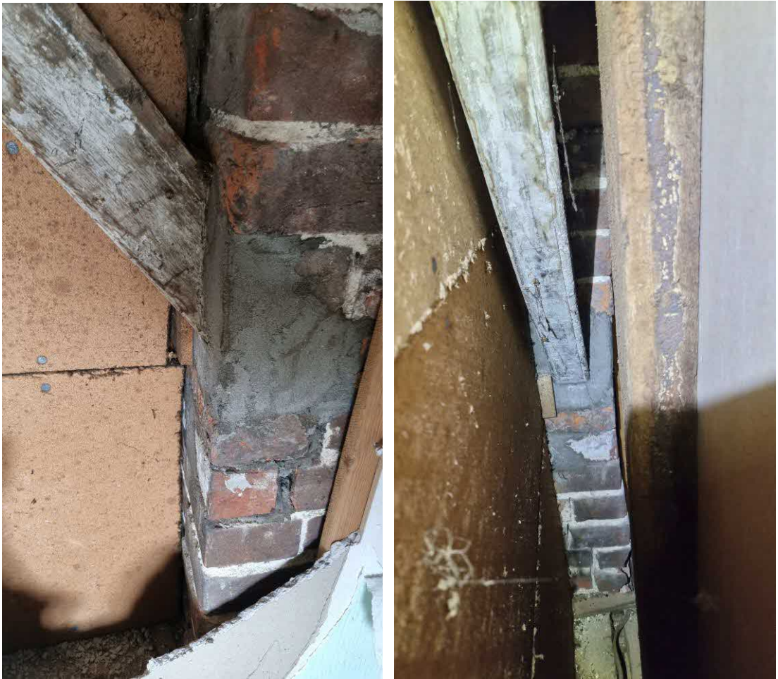
Fig.13: Timber brace appears to have been inserted into a brick wall with modern cement. The brace is one of pair located in a wall on the first floor. The cement may be a repair.
