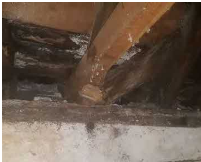
Showing rotten valley boards and wall plate
