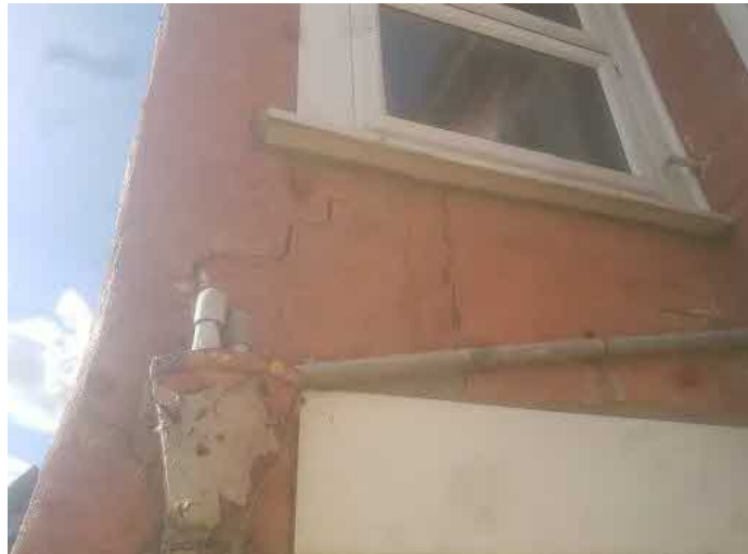
Showing wall damage on Northeast Elevation
