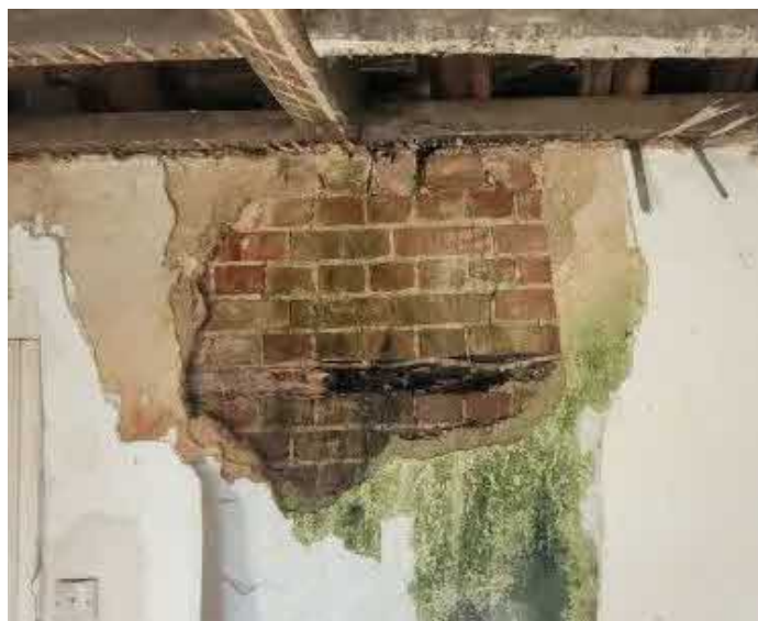
Showing wall cracking and moisture ingress
