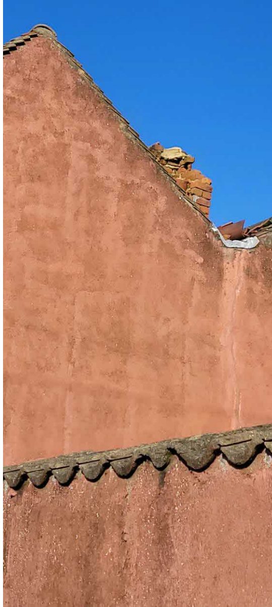
Photograph 5B Showing partially collapsed chimney in valley.
