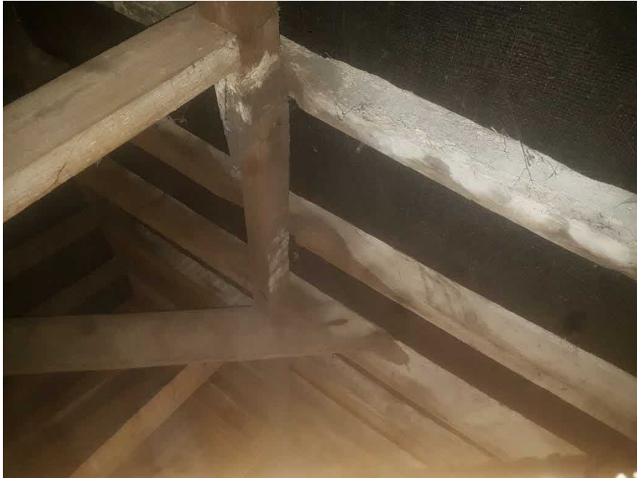
Photograph 8 Showing decaying rafters.
