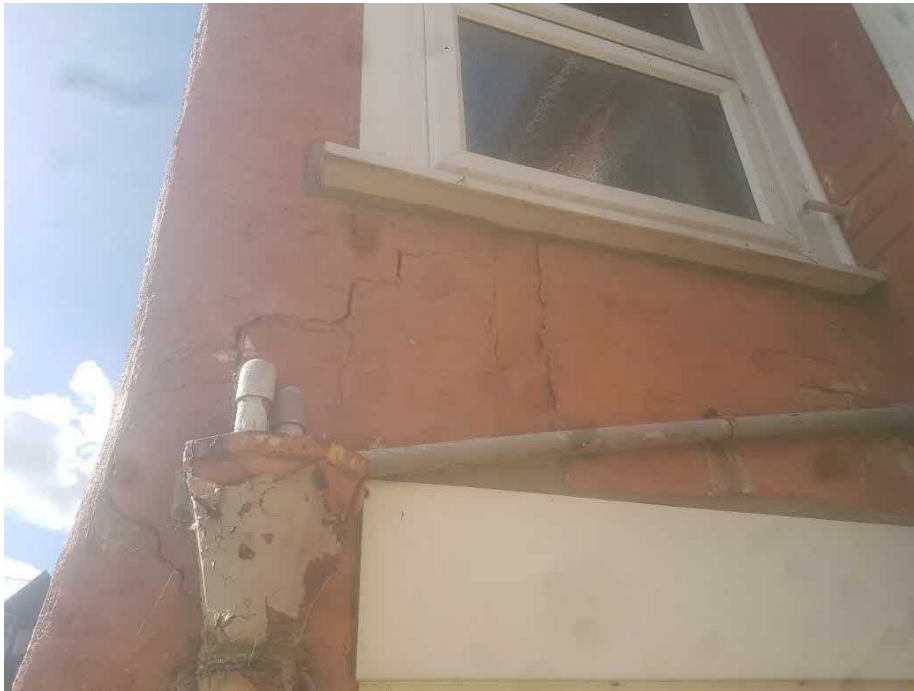
Photograph 6 Showing wall damage on Northeast Elevation
