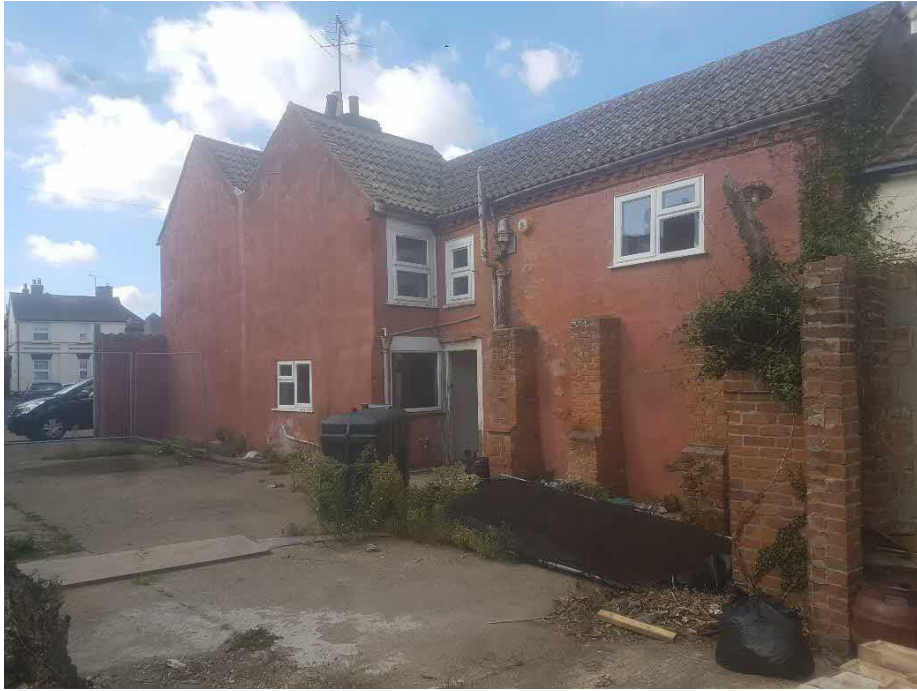
Photograph 2 Showing openings in walls on & Southeast Elevations.
