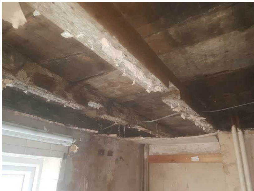
Photograph 34 Showing deep notched mid span in floor joists.
