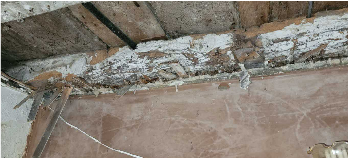
Photograph 20B Showing rotten joists over sitting room
