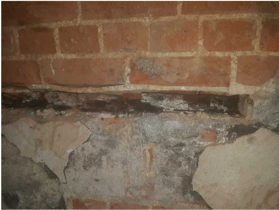
Photograph 25 Showing rotted & disintegrated timber in Study side external wall & gap left in wall.
