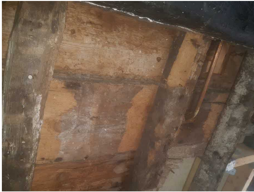
Photograph 35 Showing rotten floor joists and boards over kitchen.
