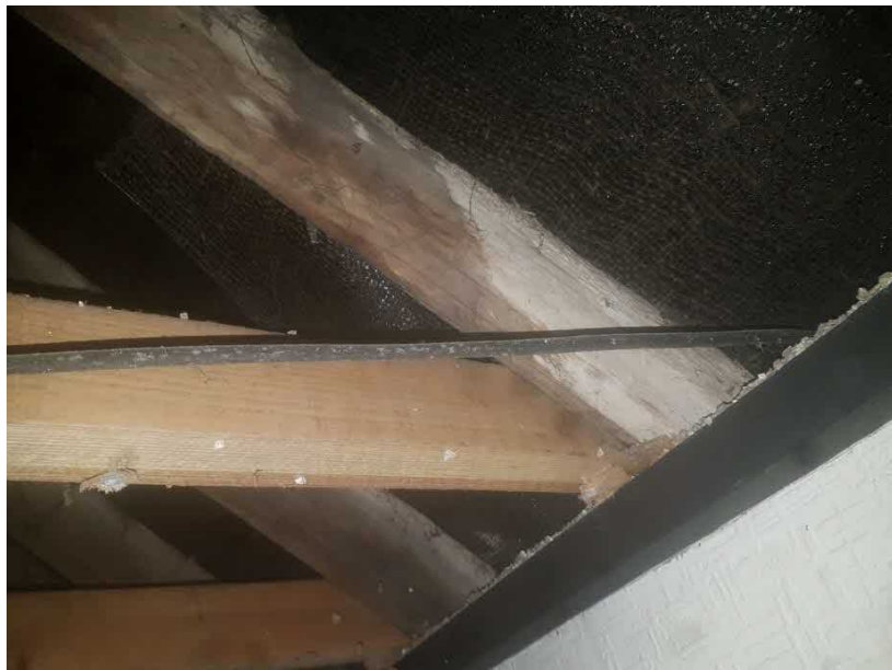
Photograph 9 Showing decaying rafters
