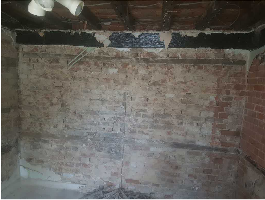
Photograph 24 A Showing timbers embedded in rear internal study wall & poorly bonded masonry
