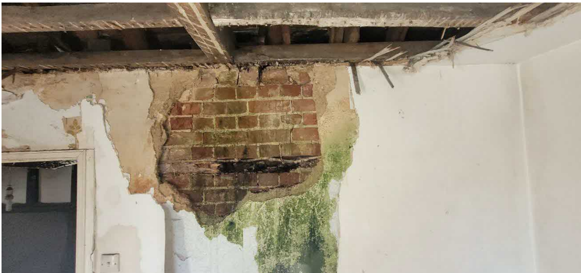
Photograph 11 B Showing wall cracking and moisture Ingress
