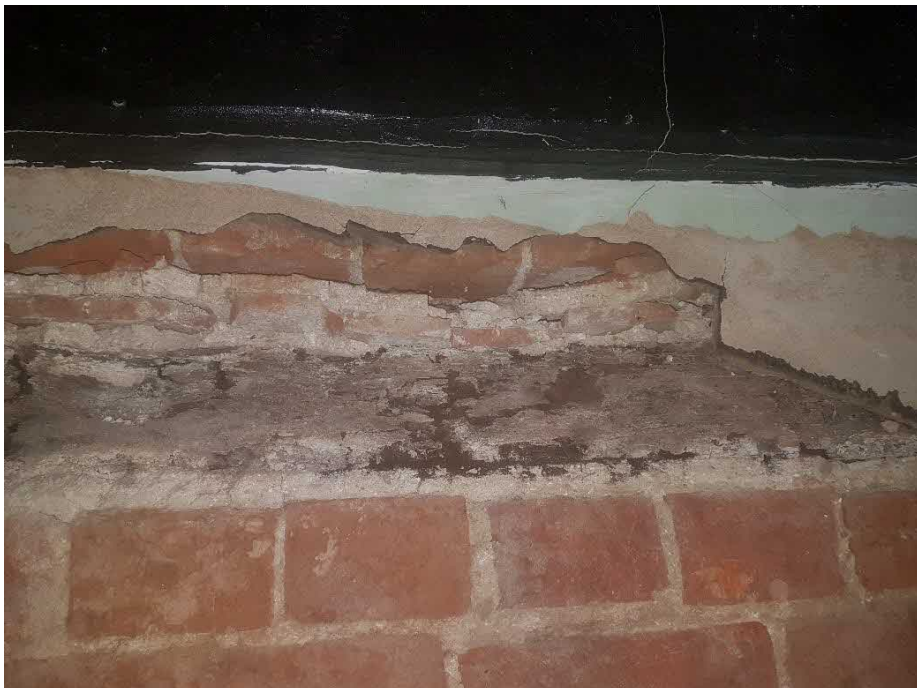
Photograph 26 Showing rotten embedded timber in external side wall in Study
