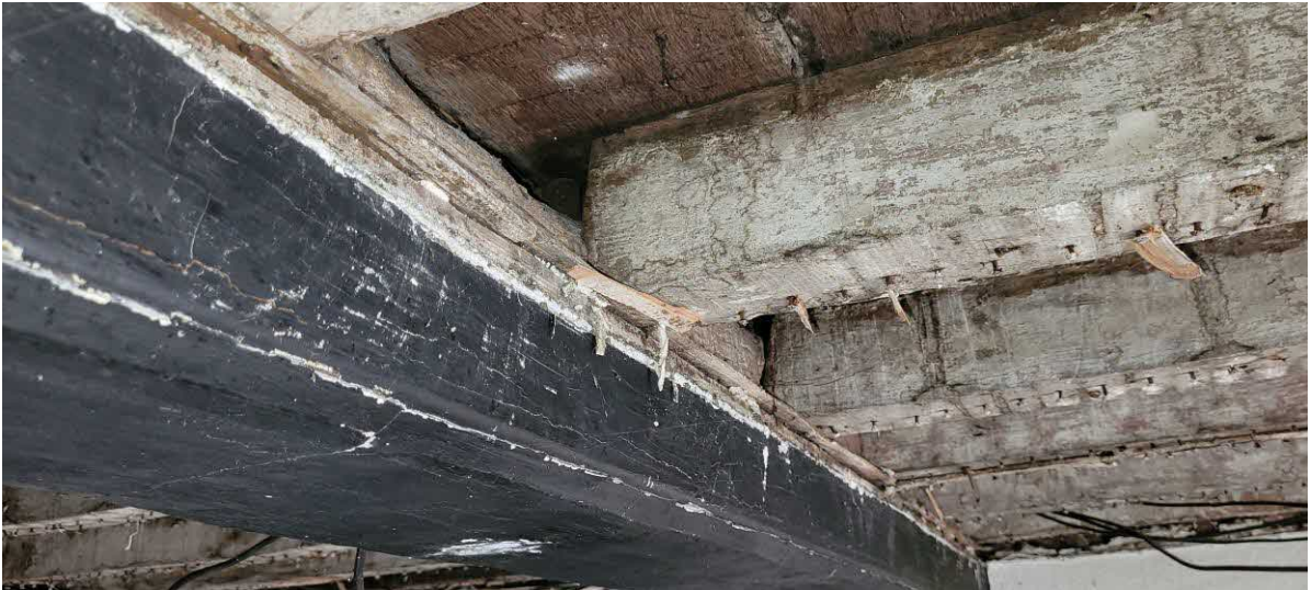
Photograph 21 B Showing joists with insufficient bearing on spine bressummer beam.
