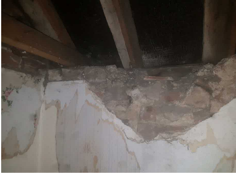
Photograph 15 Showing rotten wall plate and loose masonry.
