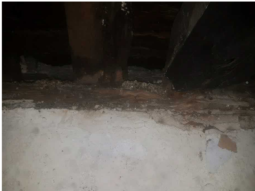
Photograph 14 Showing rotten wall plate.
