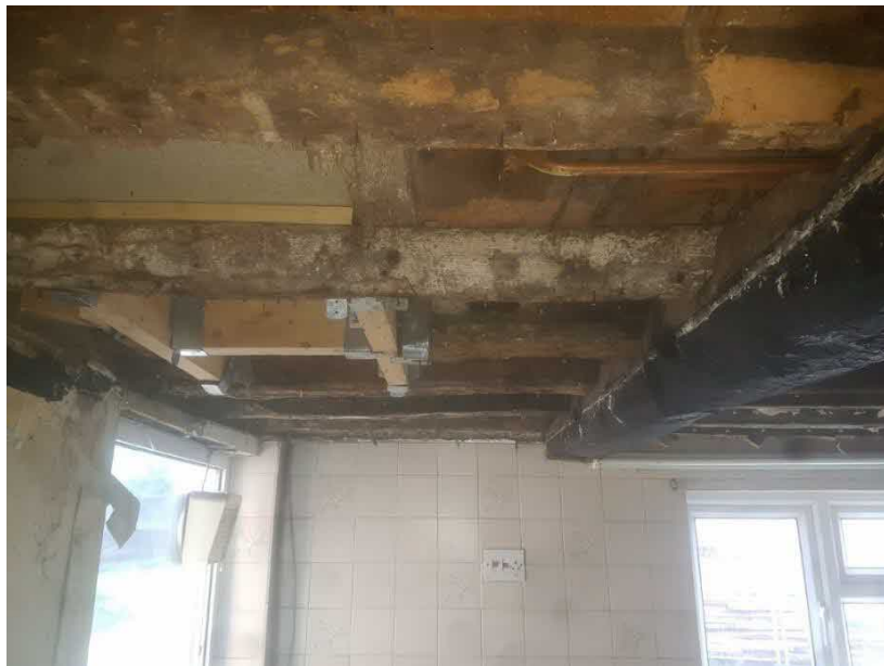
Photograph 32 Showing rotten floor joists over kitchen.
