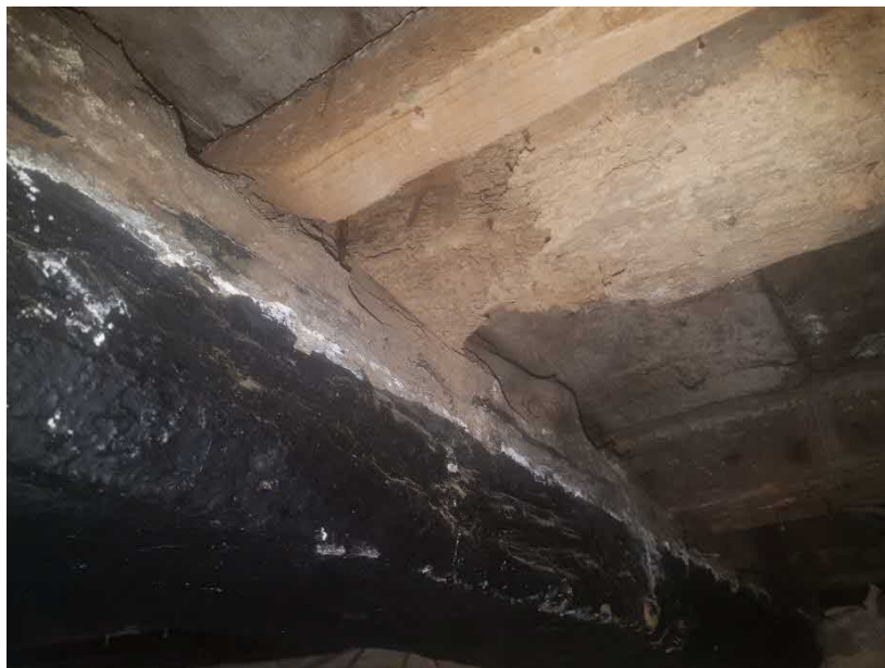
Photograph 30 Showing badly deteriorated joist and timber beam over kitchen
