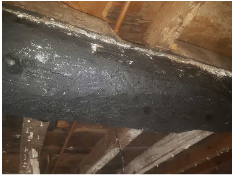
Photograph 31 Showing deep notch in timber beam that supports the floor over the kitchen.
