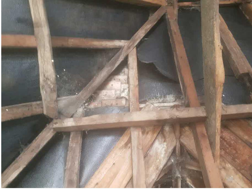
Photograph 12 Showing missing felt and rotten timbers.
