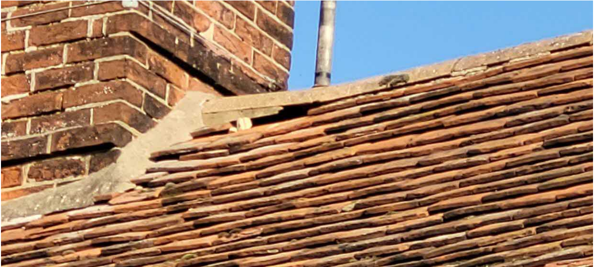
Photograph 7B Showing distortion of the main front Chimney Stack
