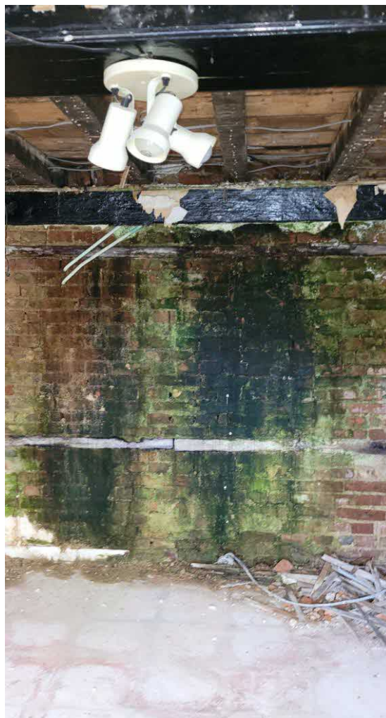
Photograph 24 B Later photo of same wall shown in Photo 24 A above – showing wall saturated after chimney collapse.
