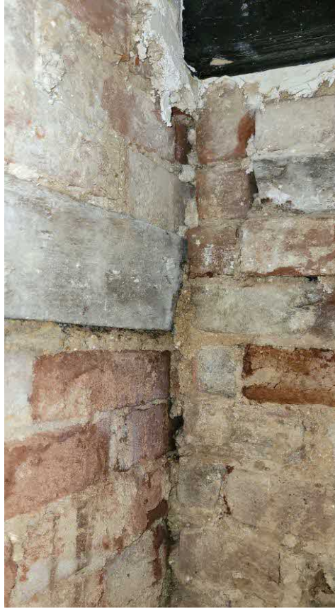
Photograph 27 Showing de-bonded masonry at internal wall junction
