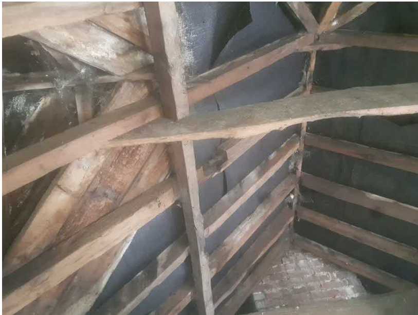
Photograph 13 Showing sagging rafters & collars
