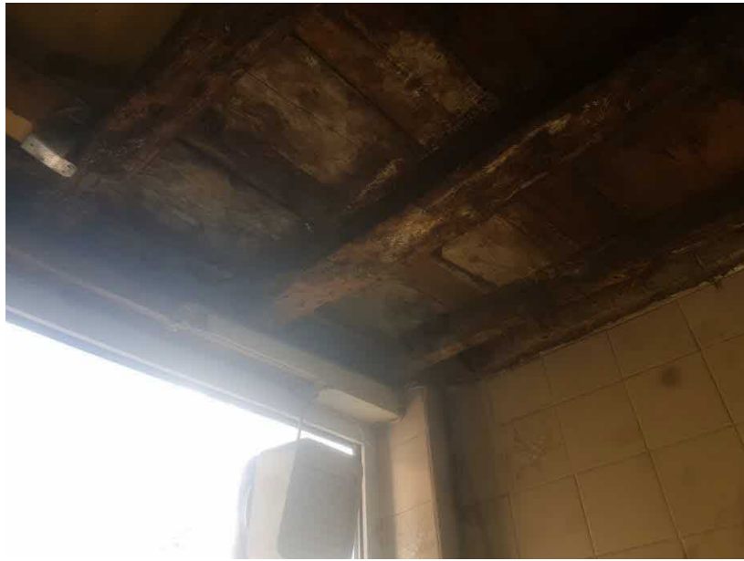
Photograph 33 Showing rotten floor joists over kitchen & no buttress return to external wall at window.
