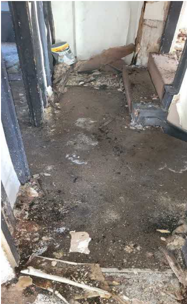
Photograph 18A. Showing area where Floor appears potentially Unsafe.
