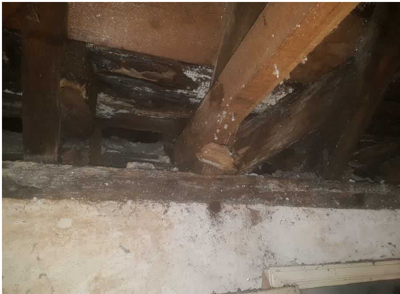
Photograph 16 Showing rotten valley boards and wall plate.
