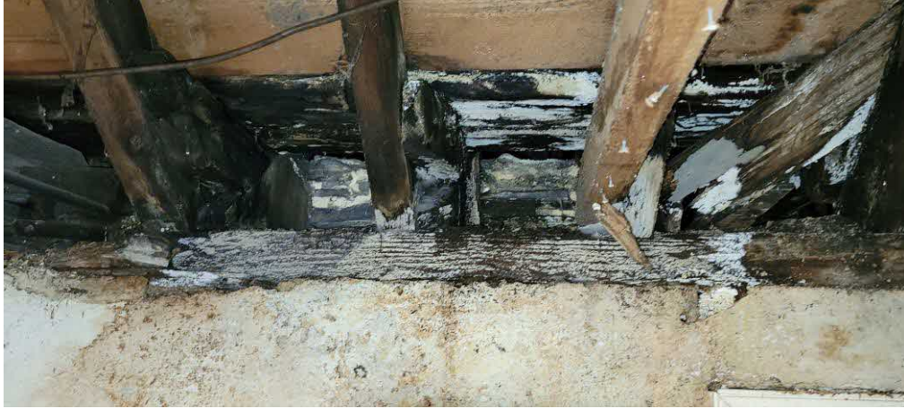
Photograph 17 Showing rotten valley boards and wall plate.
