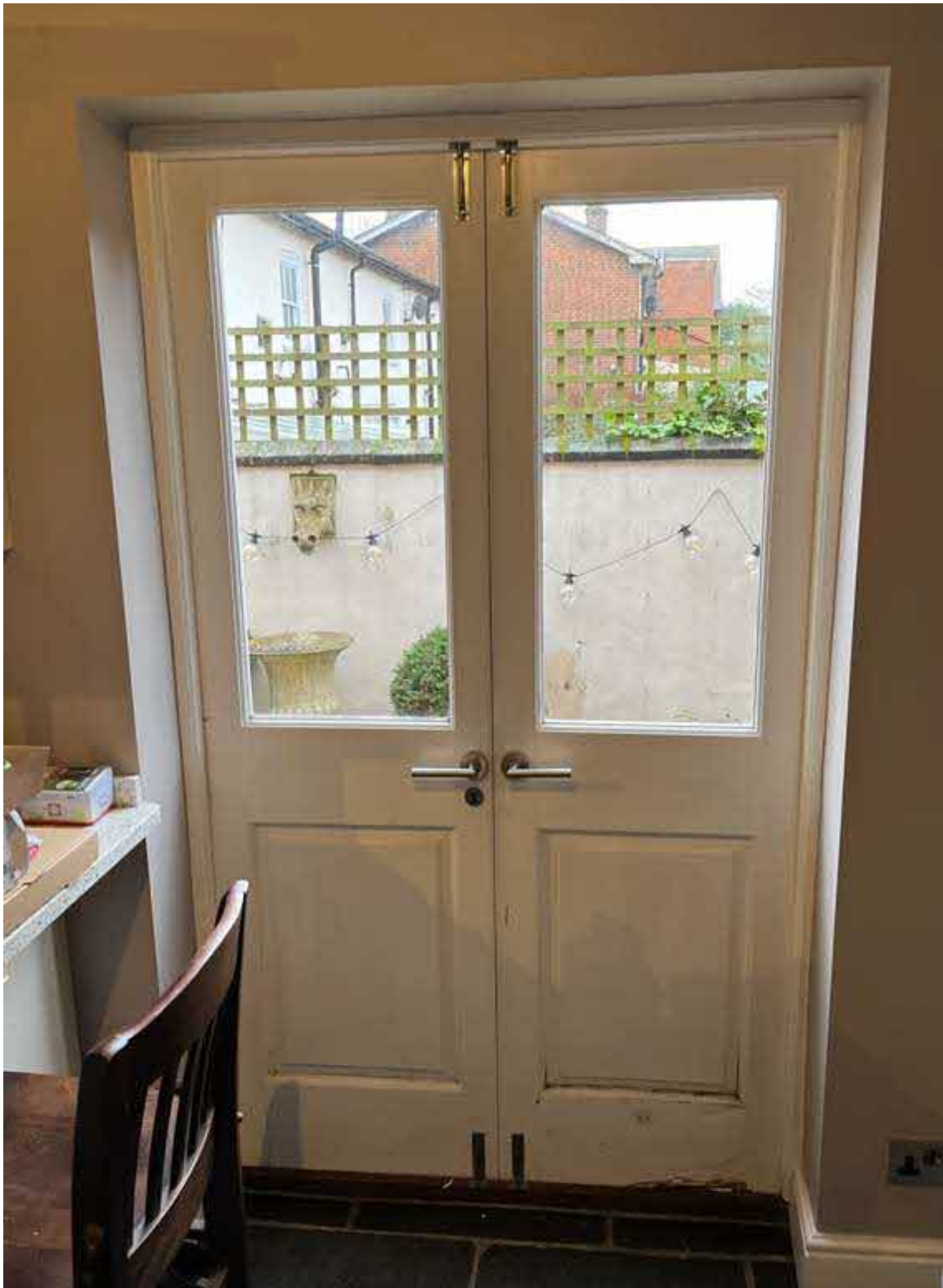
Fig. 2 –Internal view of existing rear French door. Note damage of door.
