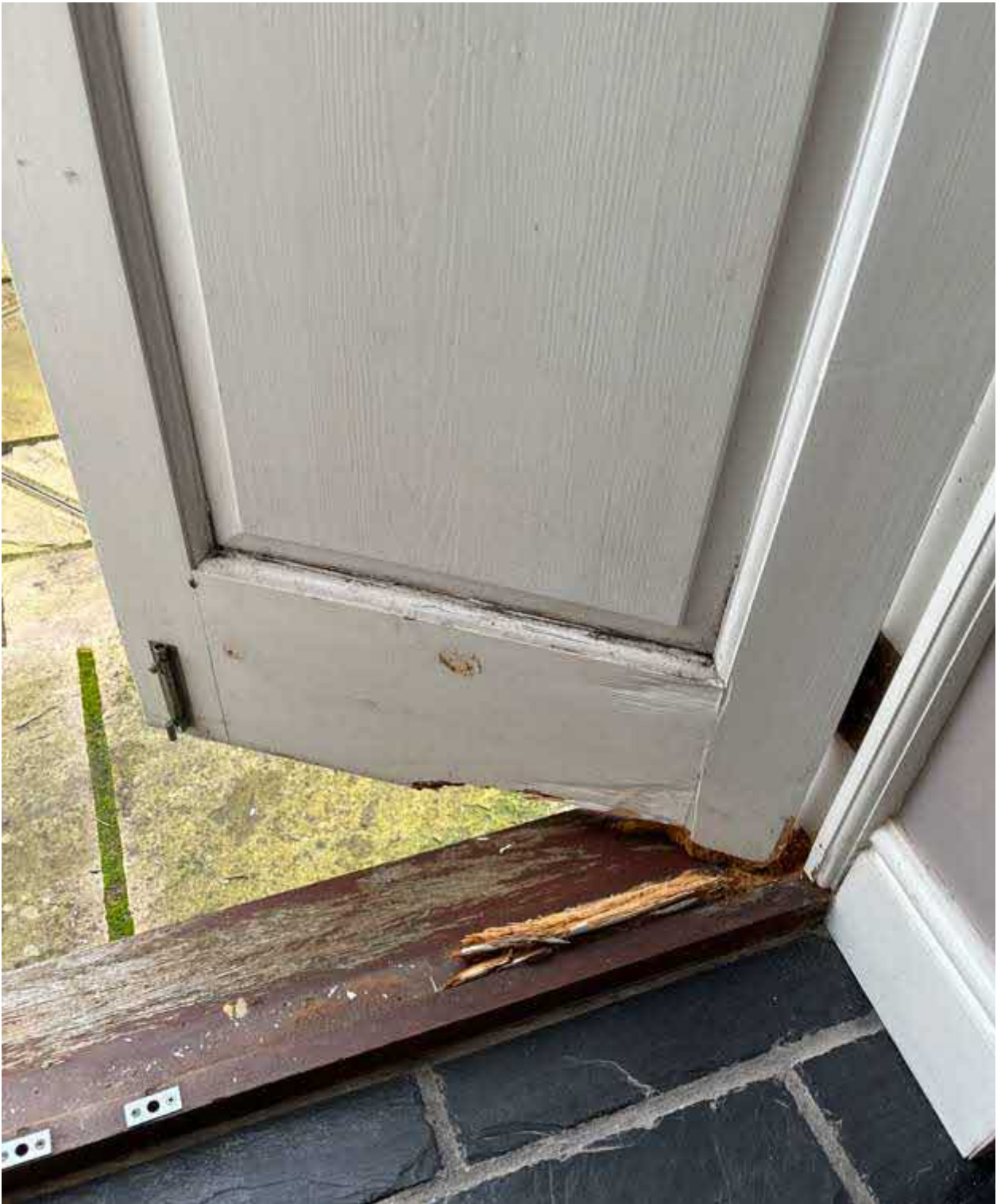
Fig. 3 –Damage to french door due to moisture ingress.
