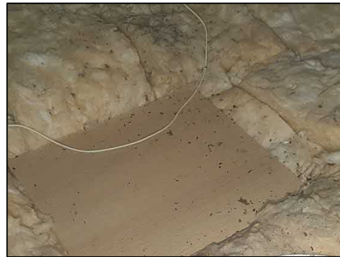
Figure 4: Droppings in roof void.
