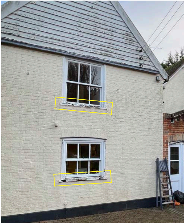
Photograph of north elevation showing both windows requiring repair.
