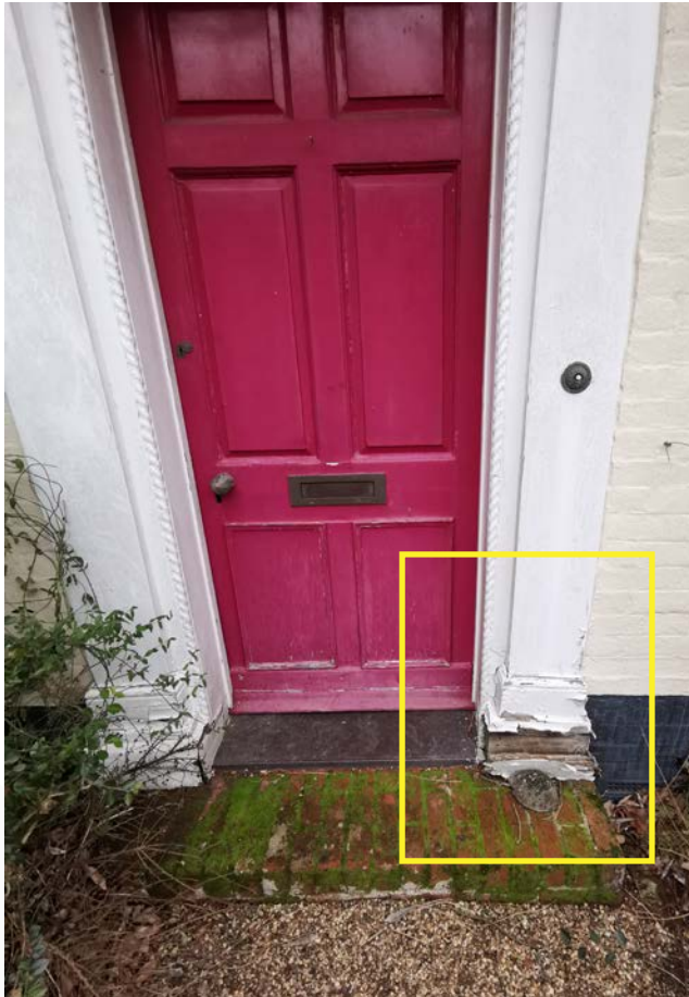
Photograph showing rotten pilasters framing the front door.
