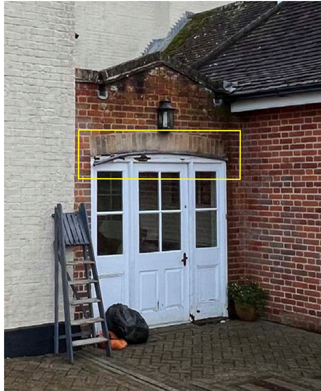
Photograph of entrance door requiring repair.
