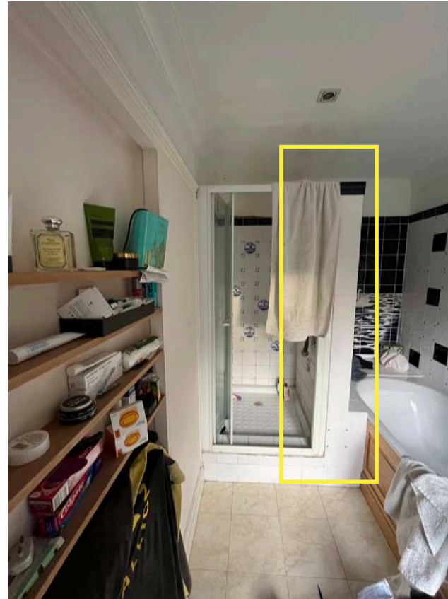
Photograph of shower built into the cubicle formed by the stud wall addition.
