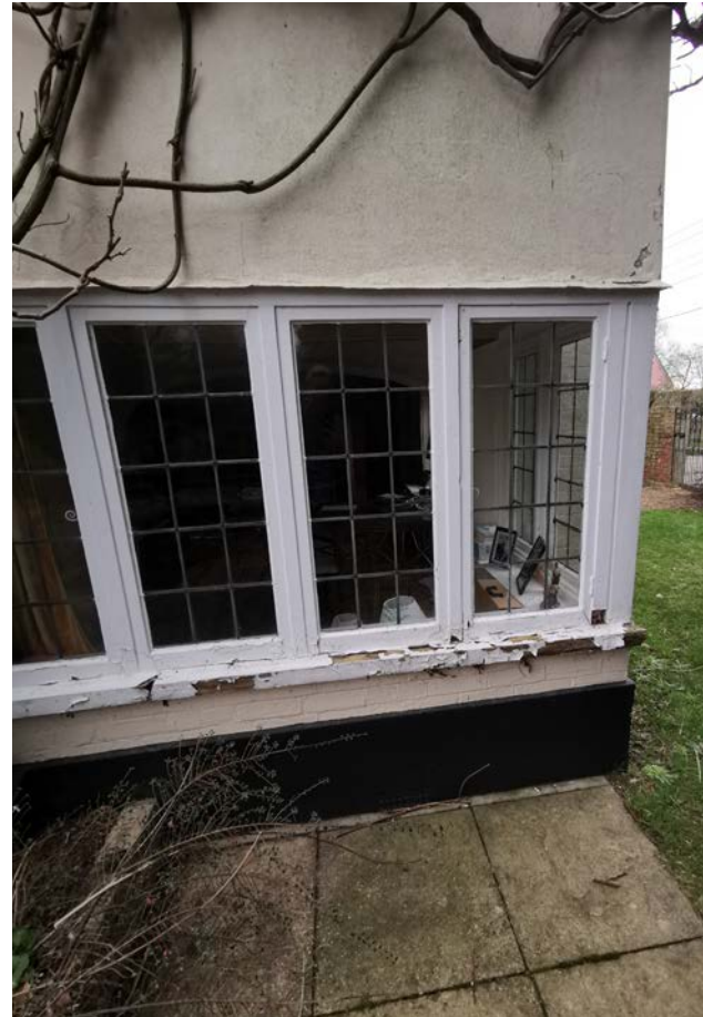
Photographs showing rotten cill on corner window to the west and south elevations. Repairs required to cill and casements, and openings to be re-established.
