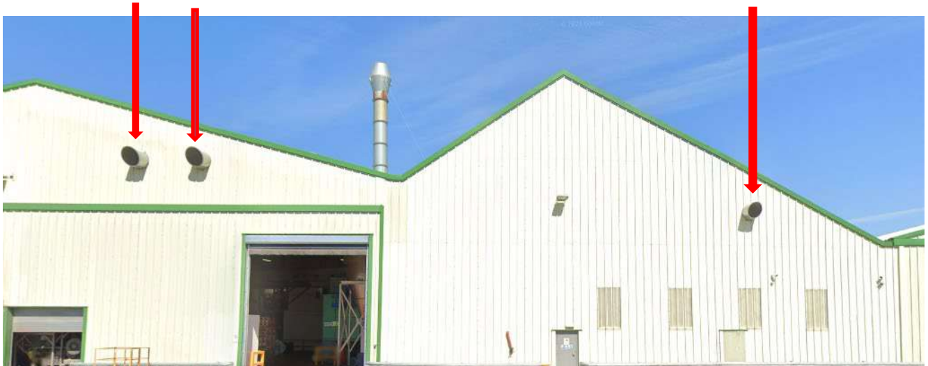
Air Movement exhaust fan Muesli line
