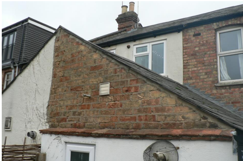
External view of rear structure highlighting the additional skin of blockwork terminating at eaves level
