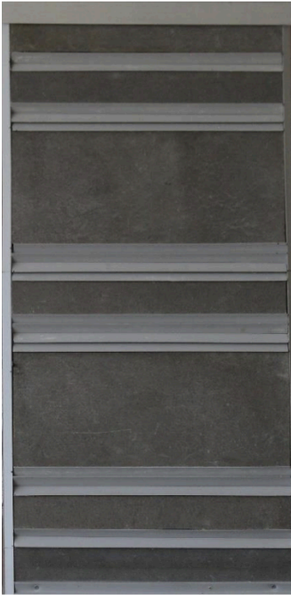
Steel rails and Cement Particle board
