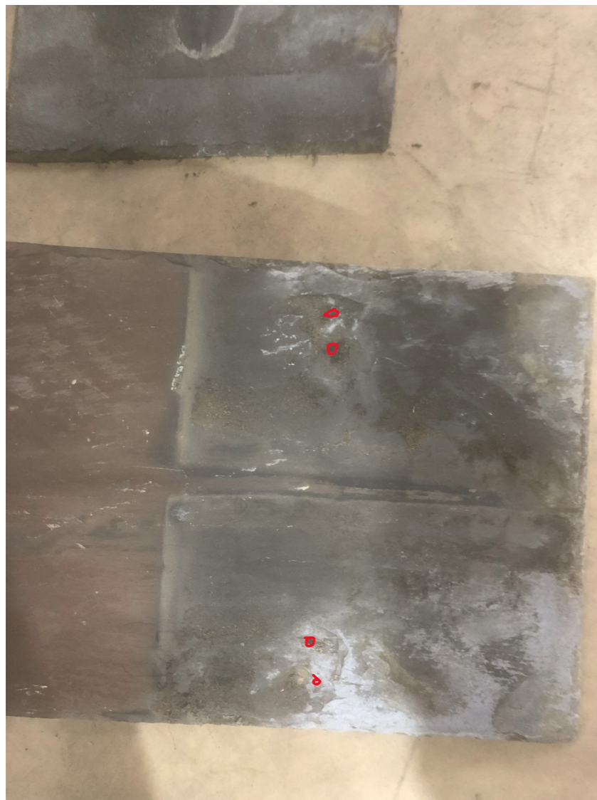
Existing Welsh slates with multiple holes
