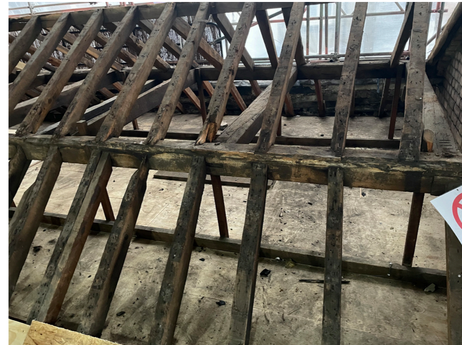
Defected and splitting rafter ends, seen throughout roofs 5 & 6
